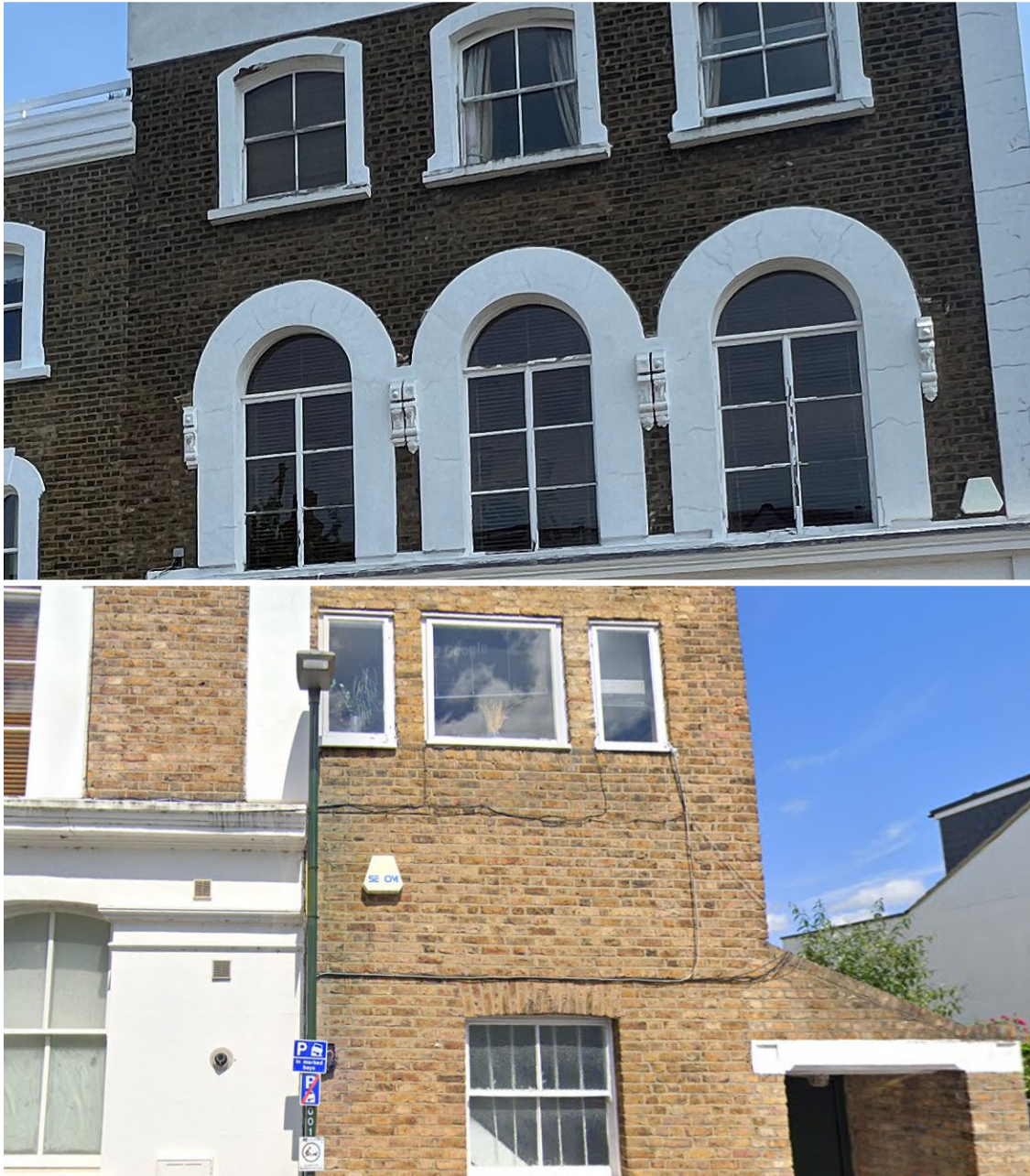
Illustration 6: The existing windows are in a poor state of repair and – in the case of the three first-floor windows on the side elevation – are considered to detract from the building’s appearance.
