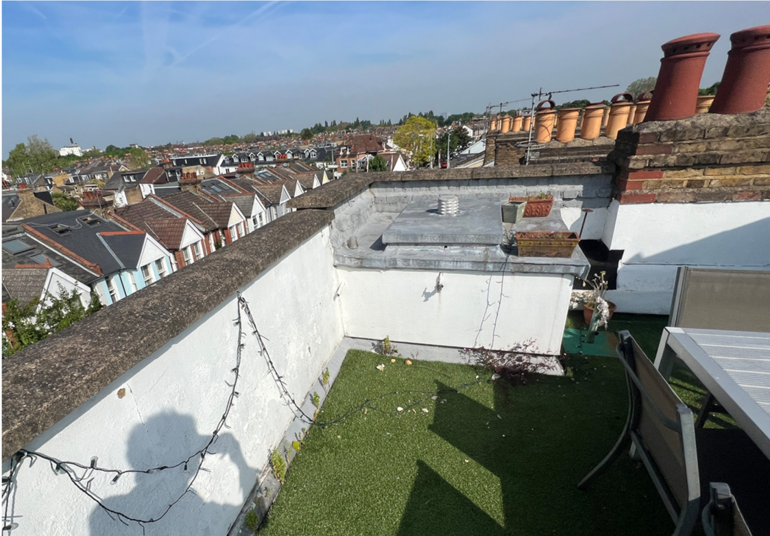
Illustration 8: the proposed condenser units will not project above the top of the existing parapet walls of the roof terrace and replace an existing (redundant) water tank.
