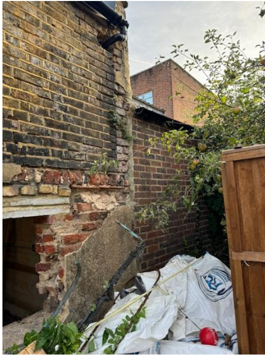
Image 2. View onto the damaged wall from existing building site at 15 Springfield Road, TW11 9AP.
