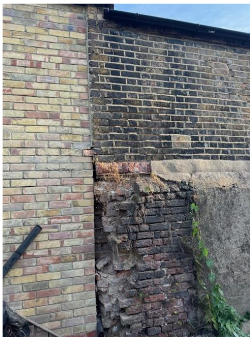
Image 1. View onto the damaged wall from 13 Springfield Road, TW11 9AP garden.
