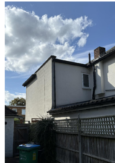
PIC 03 showing no windows at FF No 40
