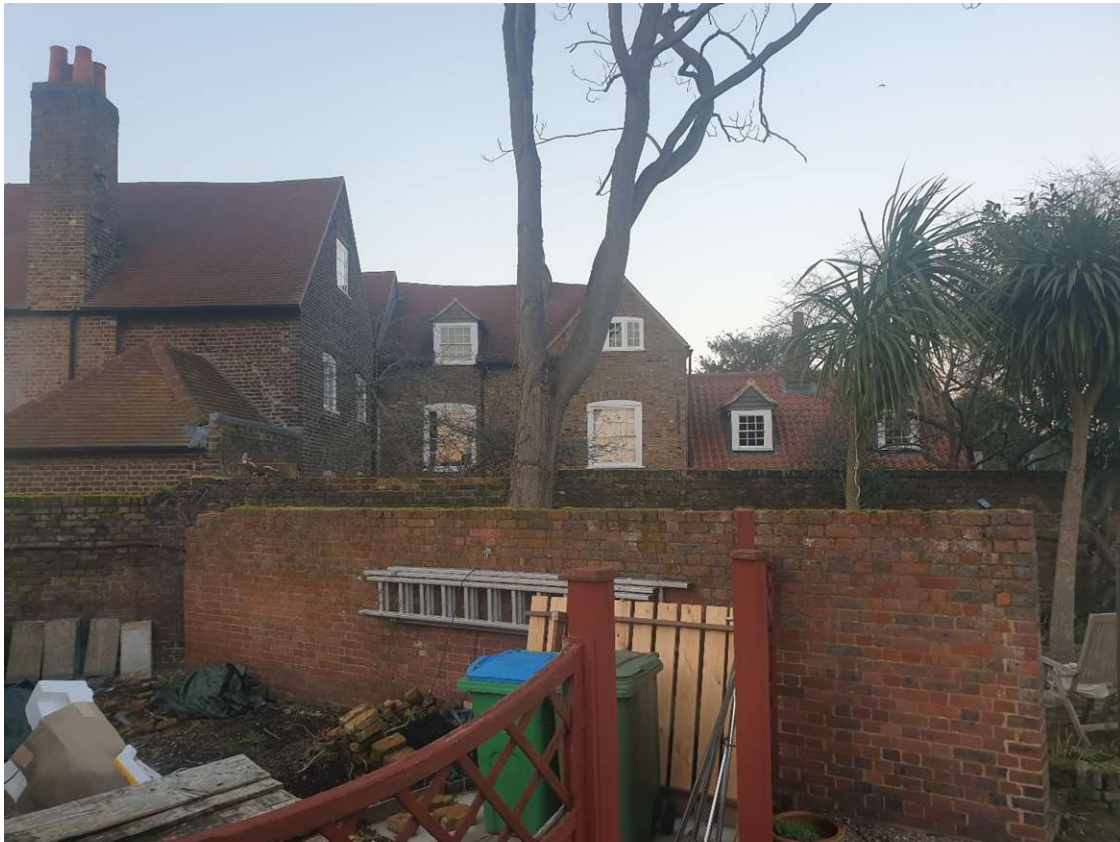
Figure 4 – View north showing isolated stretch of red brick garden wall built between the wars
