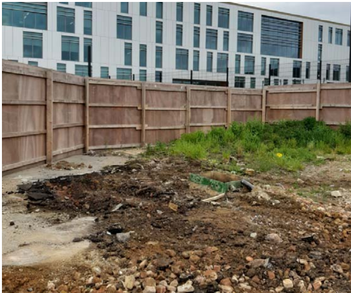
Chamber location to be removed, following oversight clearance and removal of protective mesh
