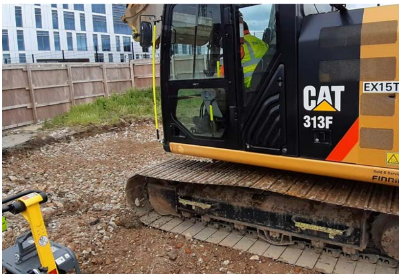
Another layer fill tracked level prior to compaction with large plate compactor on 20.05.21
