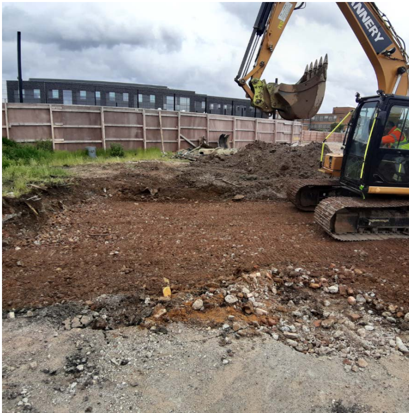
Machine levelling next layer of fill using tracks prior to compaction using large plate compactor on 20.05.21
