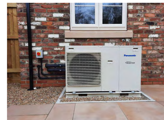
ref.27: Air Source Heat Pumps
