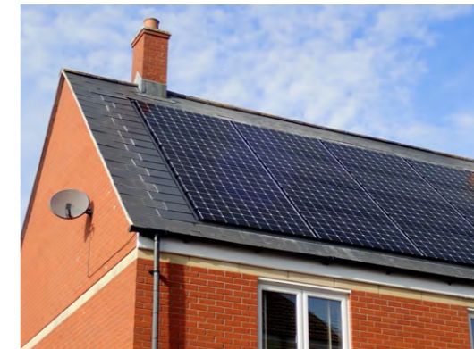
ref.26: Solar Panels
