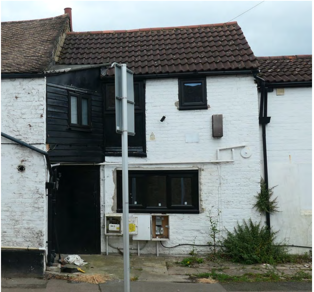
Photo 13: The east (May Road) elevation of the heavily altered/partially rebuilt mid-late C19 two storey extension with a rear catslide roof.
