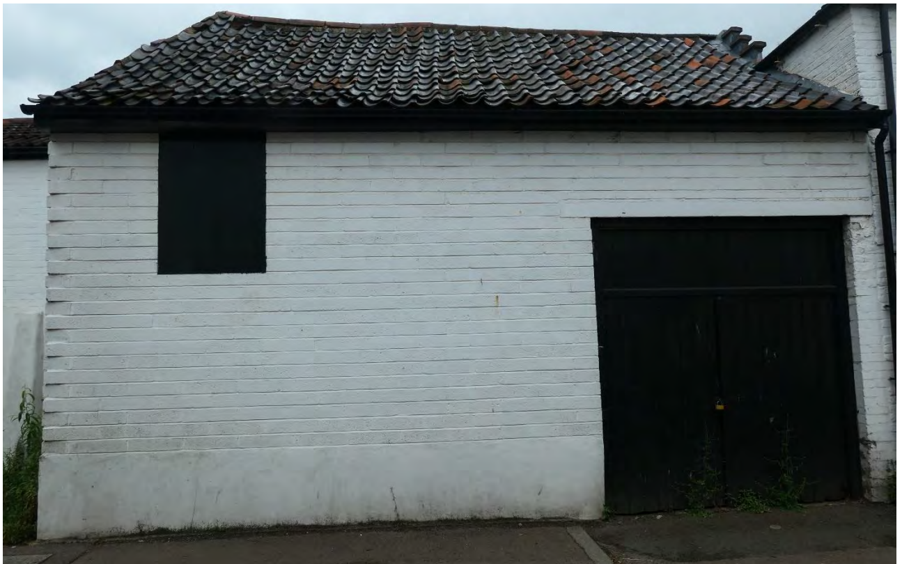
Photo 20: Almost all of what can be seen of the partially rebuilt mid-late C19 two storey extension from May Road is a modern reconstruction, executed to a rather poor standard, as evidenced in the brick 'toothing' at the southern corner.
