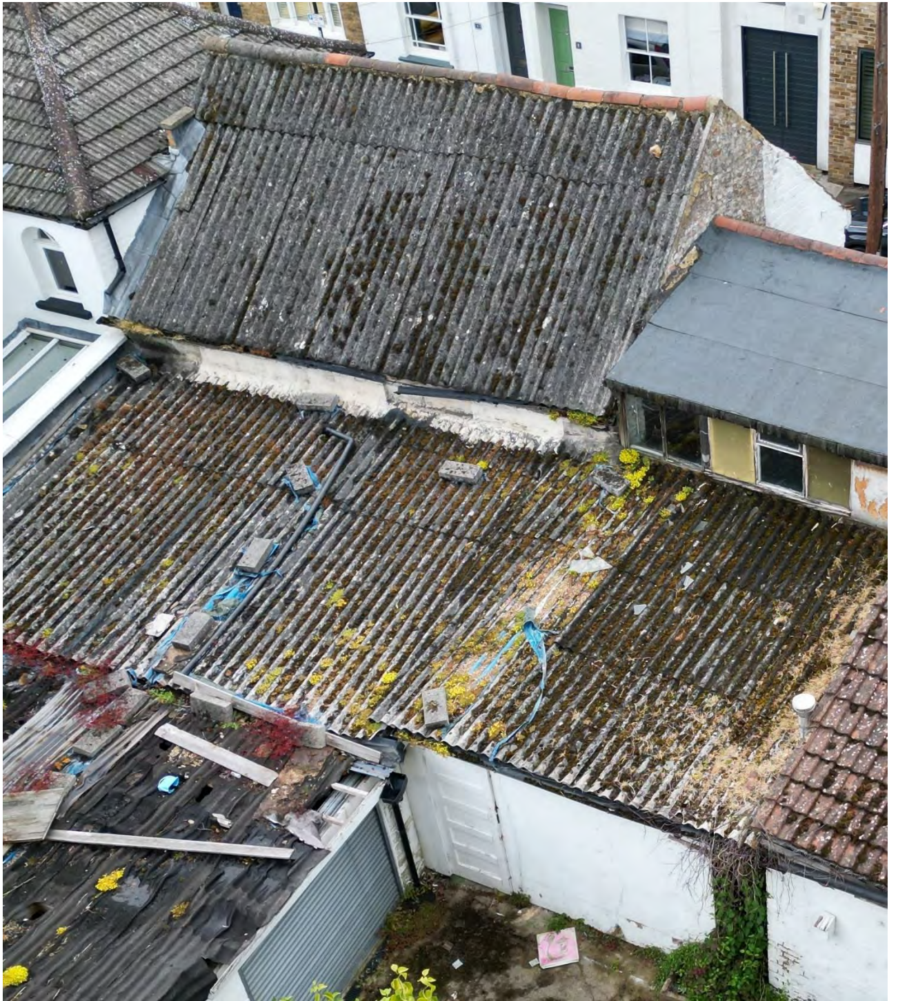
Photo 22: Almost all of what can be seen of the partially rebuilt mid-late C19 two storey extension from May Road is a modern reconstruction, executed to a rather poor standard, as evidenced in the brick 'toothing' at the southern corner.
