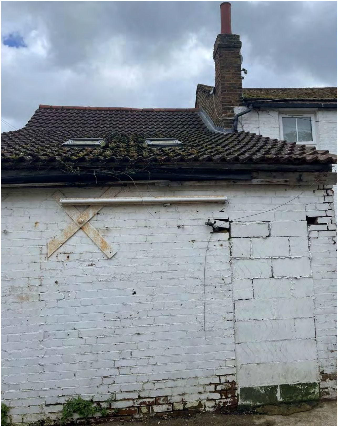
Photo 16: The back of the heavily altered/partially rebuilt mid-late C19 two storey extension with a rear catslide roof, seen from the south.
