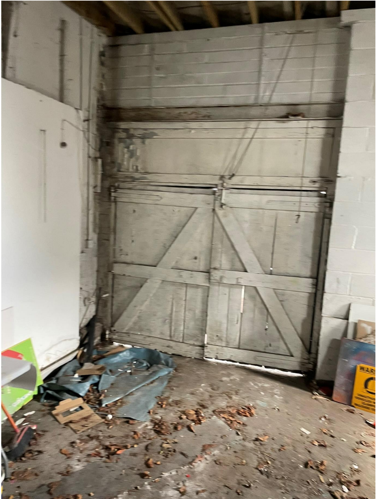
4.21 The front of the workshop along May Road appears cleaner than the back of the site but the concrete slab on the floor needs to be investigated for its structural integrity. There are cracks and depressions which highlight movement and it would need to be investigated, reduced in level and re-cast as a residential structural floor.
