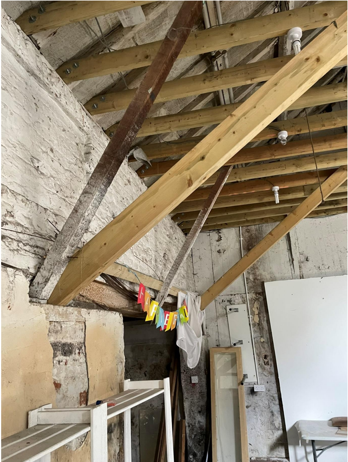
4.18 The roof has been additionally supported in several areas but without adequate wall plates which would need to be added to them. The ah hoc placement of roof supporting members would not be fit for purpose and would need to be altered or re-designed and placed appropriately within the roof space.
