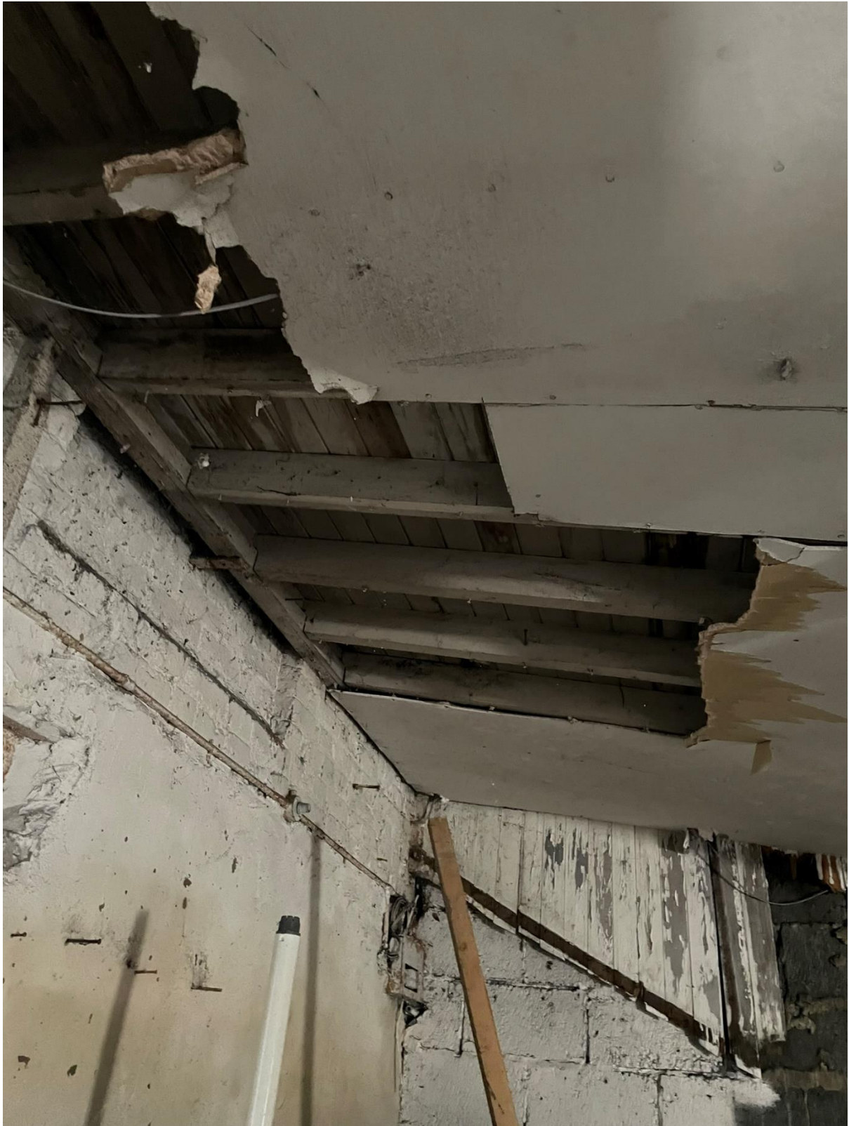
4.22 As we have seen the roof timbers are not fit for purpose and would need to be replaced. The connections to the masonry are poor and there is moisture and damp that has penetrated into the building.
