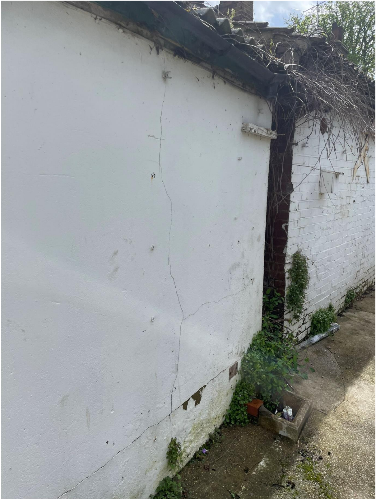
4.15 Similar to the extension façade, there are issues with moisture and damp. This is evident by the vegetation growing within the structure. The vegetation must be cleared out and the render stripped back to understand the condition of the brickwork. There are more cracks along the wall but these seem to be consistent with thermal and moisture movement.
