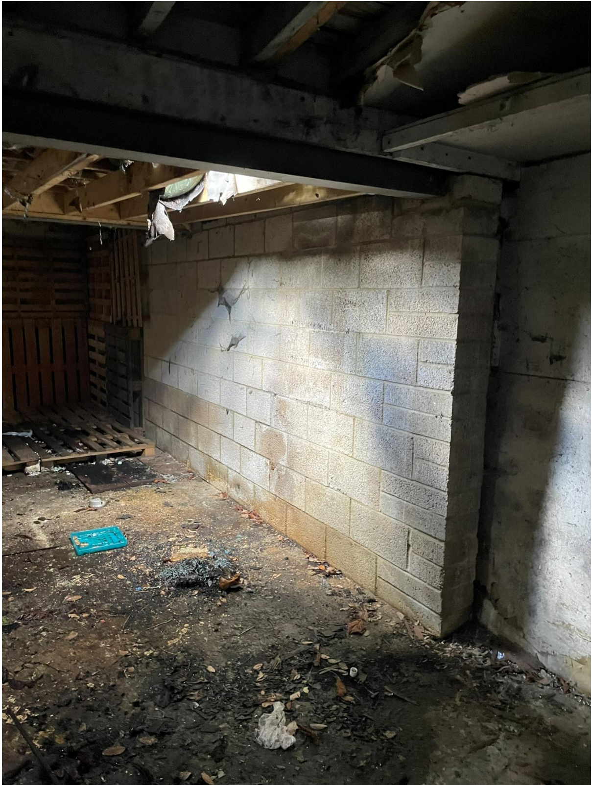
4.24 Highlighting the poor condition of the floor and the roof. There is a new masonry wall in blockwork that has been constructed. It may be supporting a wall that is failing and that should be investigated.
