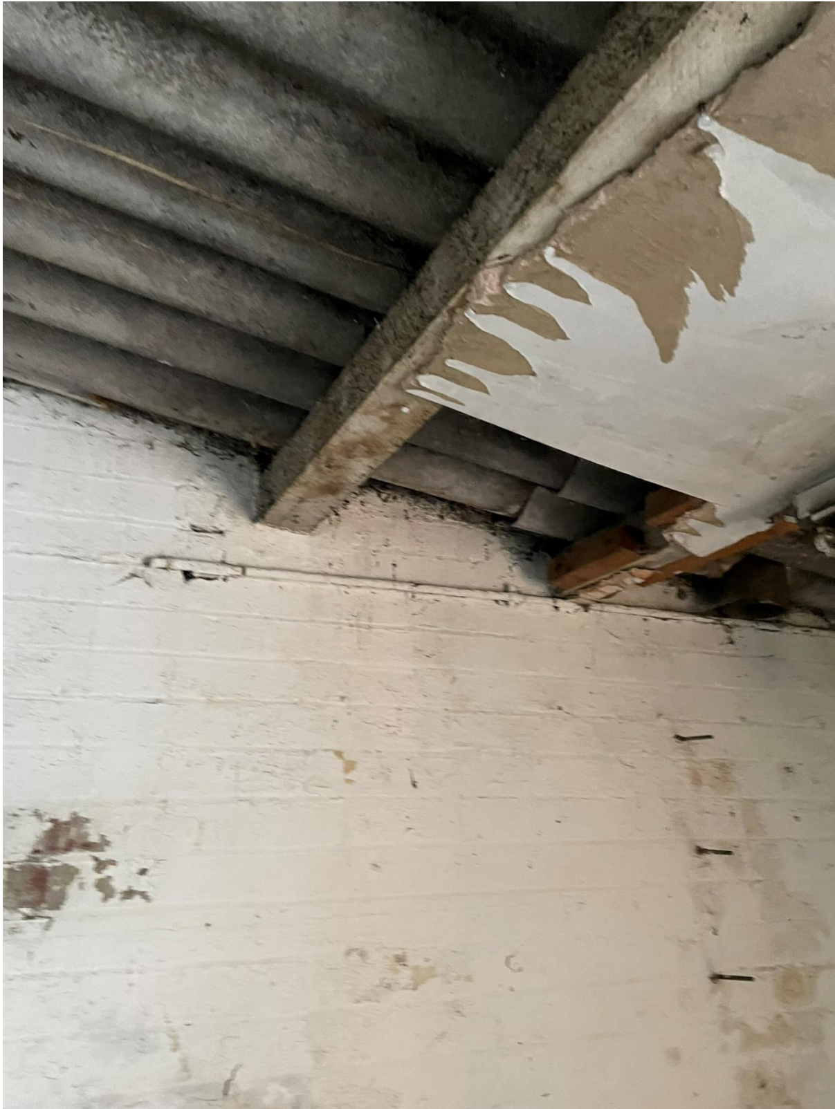
4.17 The timber along the existing roof structure needs replacing as well as the cement roof sheets which have been flagged to contain asbestos and are a hazard. Therefore, it would be recommended to replace the full extent of the roof of the workshop and garage.
