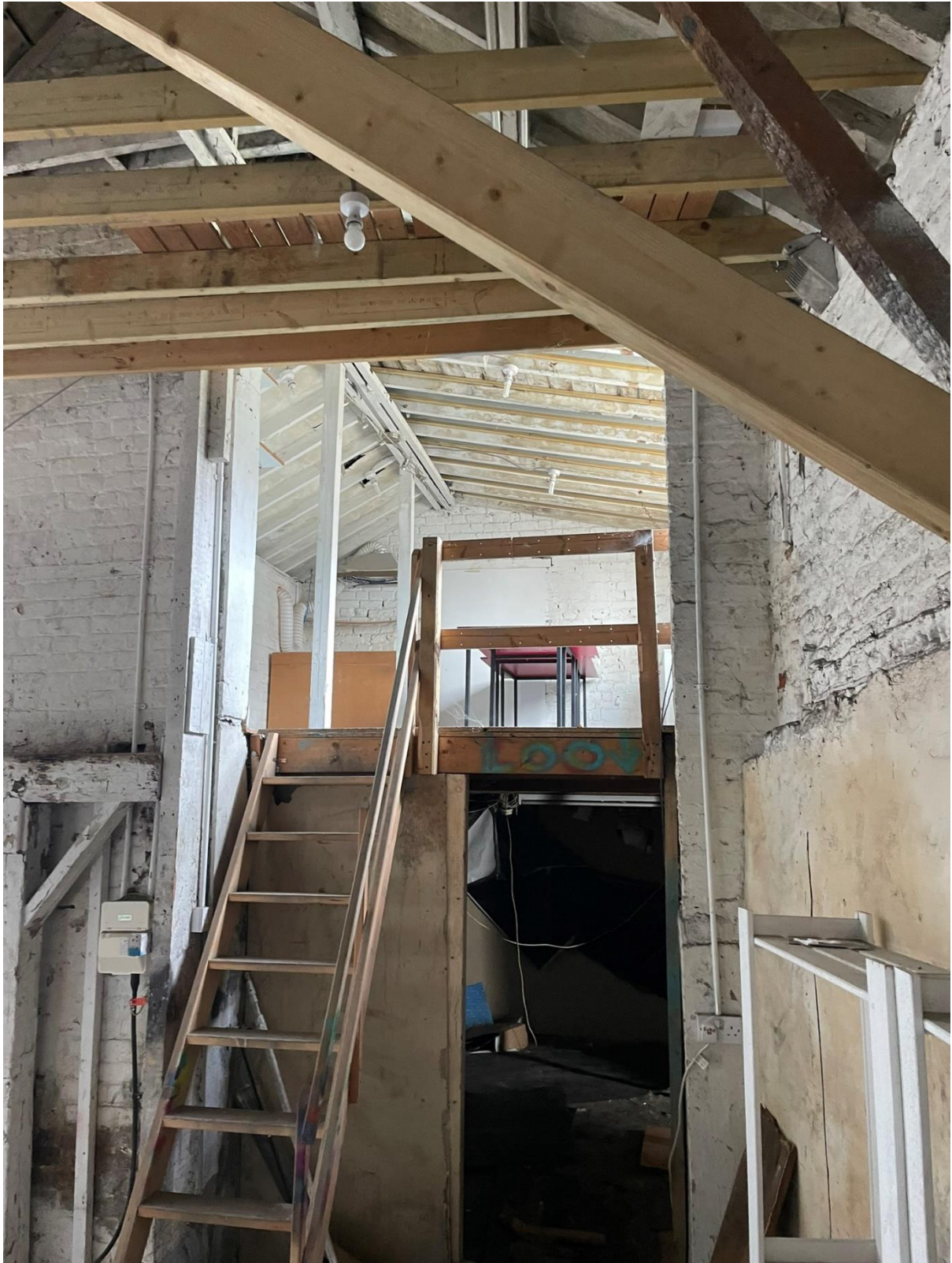
4.20 The makeshift mezzanine layer of the workshop appears to have been built without a consideration for modern load requirements. While the timbers are relatively newer than most of the roof structure, they are smaller in size and would not be compliant for a residential floor due to strength and vibration.
