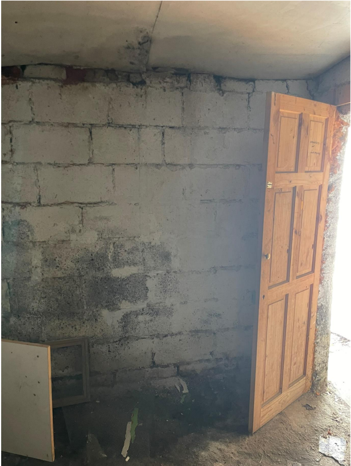
4.16 The wall is of masonry blockwork construction but there are issues with the quality and workmanship of the blockwork and the mortar. Significant work will need to be done to ensure that it is suitable for the proposed building. There is also damp and mould which may affect the structural integrity of the blocks and these will need to be stripped back and checked.
