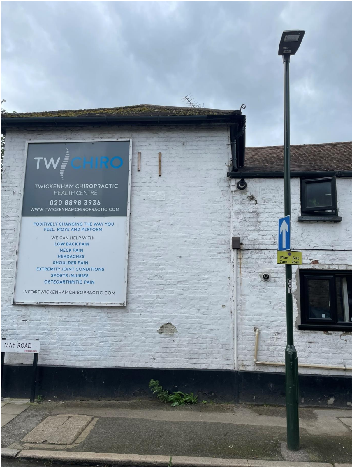
4.4 There is a visible join along the main building and the extension that was added later. The roofs have also been integrated with the main roof. The wall along the side elevation does not show any significant concerns as well.
