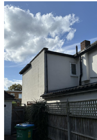
PIC 03 showing no windows at FF No 40
