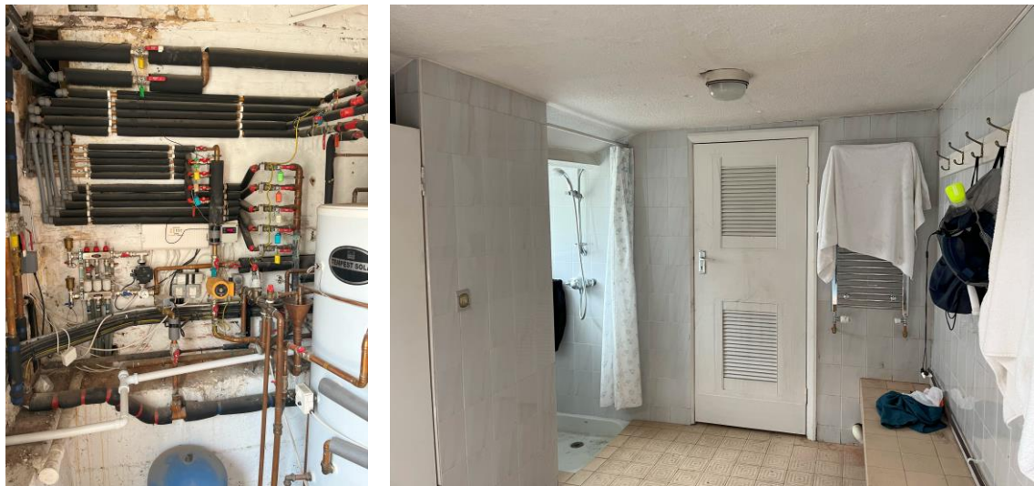
Figures 18 and 19: Internal view within the western end of the ancillary range comprising plant room and pool changing rooms
