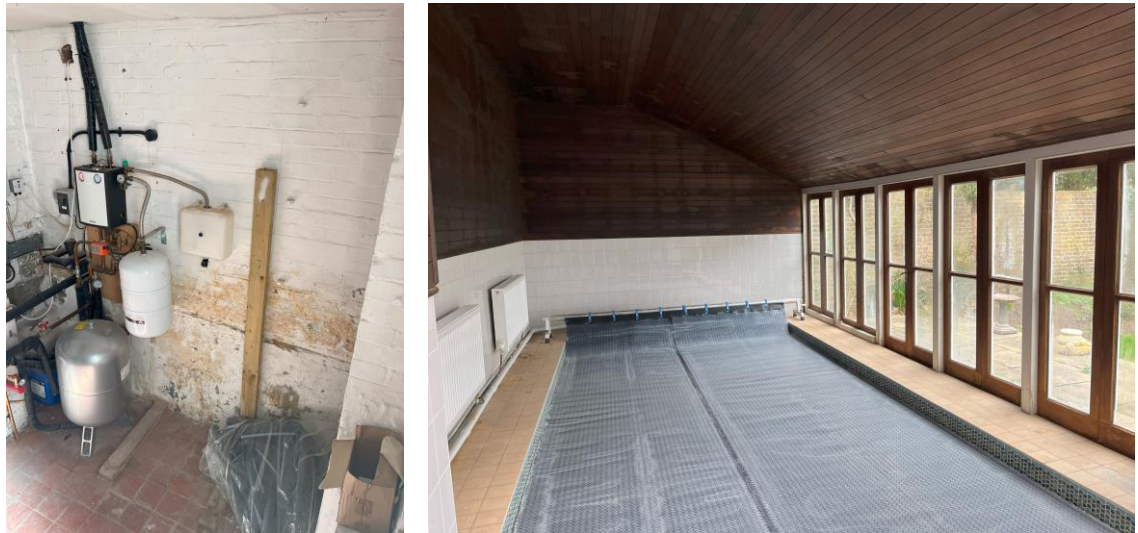
Figures 22 and 23: Ancillary plant room within the range (left) and internal view within the pool house (right)
