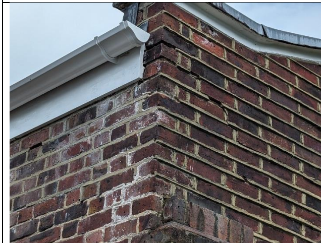
Photograph 3: Mortar gaps in the brickwork.
