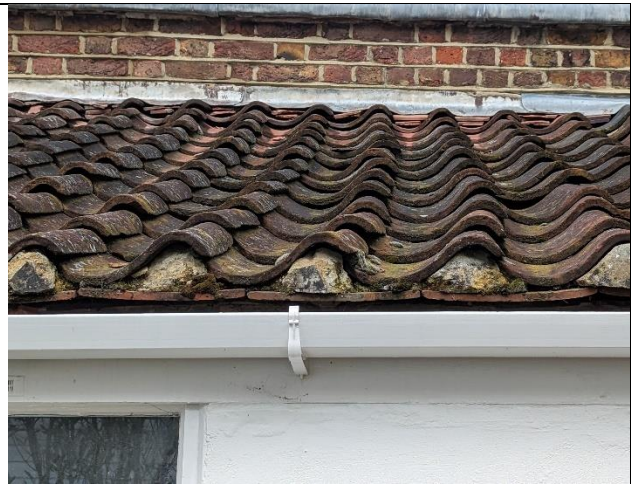
Photograph 2: Lifted roof tiles.
