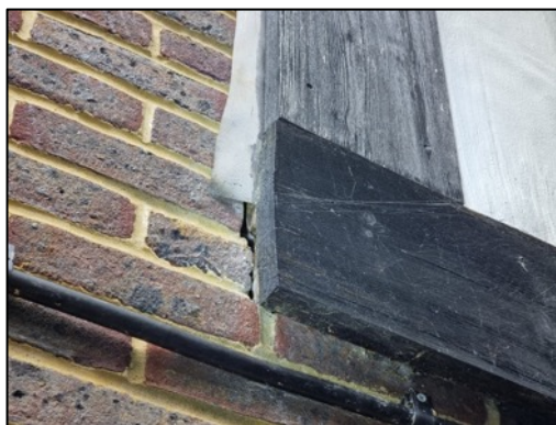
Figure 14 – gaps between the timber work and wall plate
