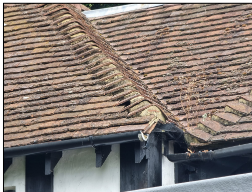
Figure 13 – missing mortar under the hip tiles on the western extension
