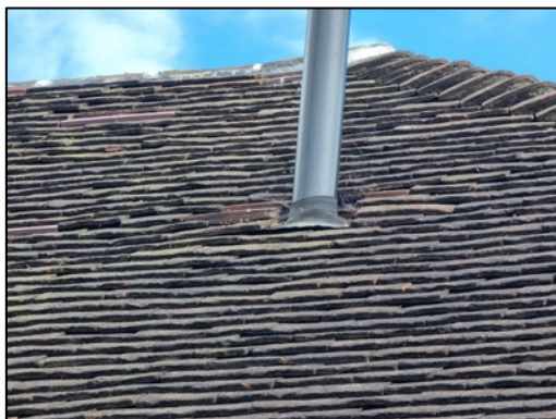
Figure 12 – lifted roof tiles on the southern roof face
