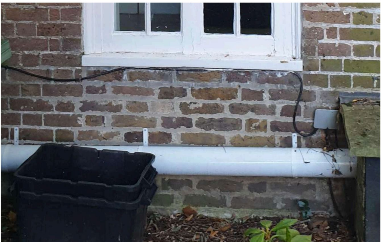
Fig 11: Image of brickwork below window on front elevation showing infill brickwork from earlier entrance door.
