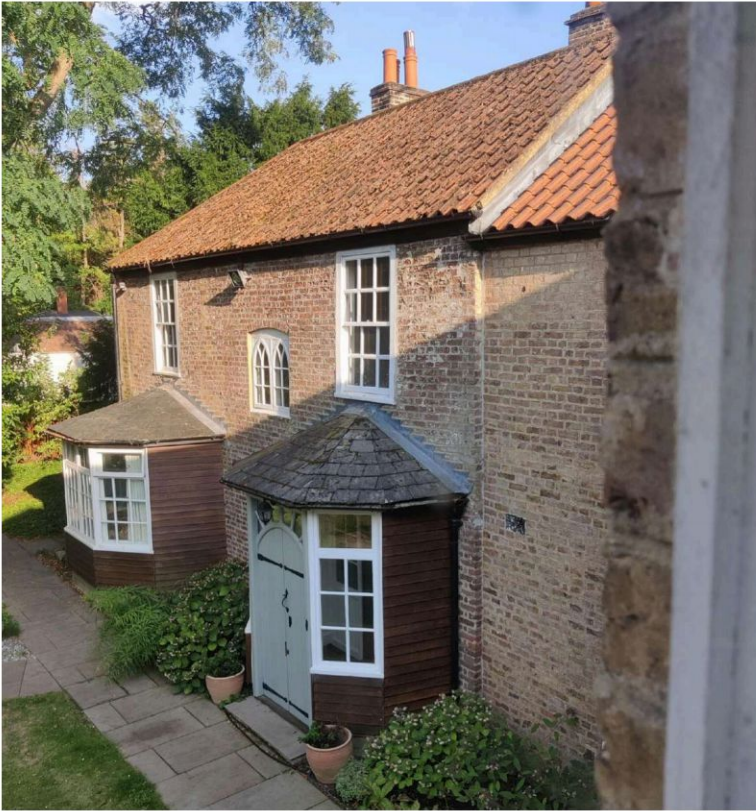
Fig 16: Side view of the modern bay structures. Note the use of slate roof which differs from the main roof and original plain tiles on Glen cottage. Further to that, the slate roof is at such a shallow angle it is only possible to weatherproof it with the use of sarking felt, a modern roofing material.
