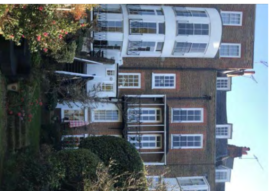
Image 1 - Before repair to upper balcony was required
