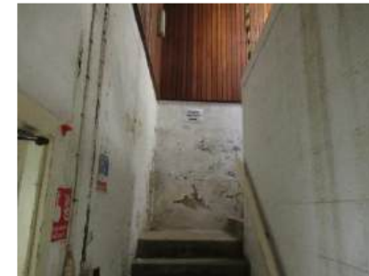
Photo 1 Water damage to right side basement stair in the main Kneller Hall west wing building (Photo taken from Jones Lang LaSalle IP, Condition Survey Report - Kneller Hall Guard House, 2020)
