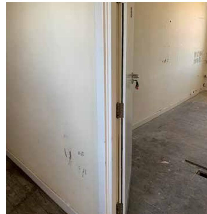
Figure 5.14 Photograph of a typical stud partition within the west wing at second floor level which is proposed to be removed Drawing produced by ADP Architecture
