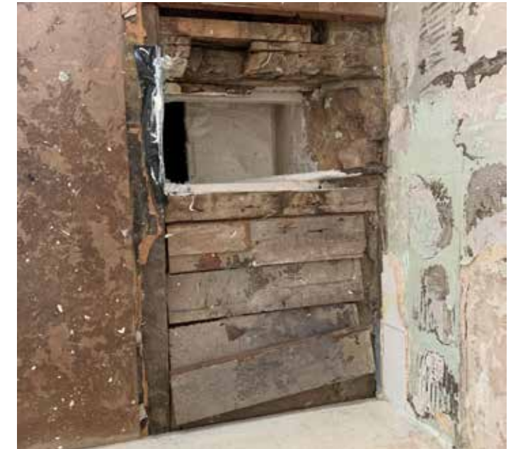
Figure 5.19 Photograph of exposed historic floorboards within the Meeting Room at Ground Floor Level
