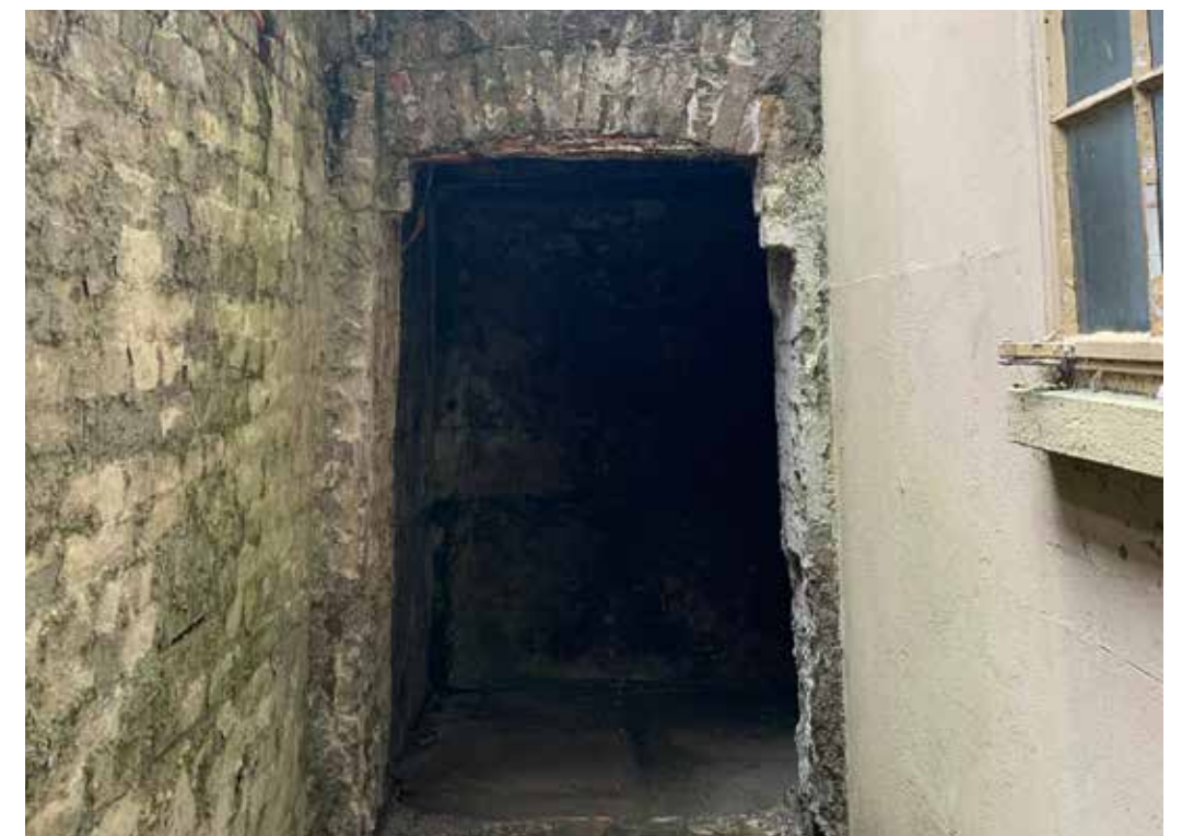
Figure 4.8 An historic external entrance survives at the rear of the basement but is in a state of disrepair
