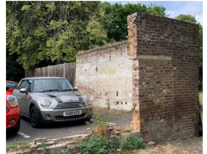
Figure 3.46 Photograph of the surviving section of garden wall. The wall is in a state of disrepair and is structurally unstable.
