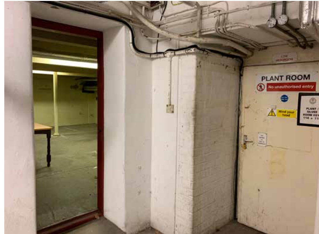
Figure 4.5 A typical corridor within the basement of the hall comprising early nineteenth-century walls which have been inappropriately fitted with exposed MEP equipment. Modern doors have also been introduced here.
