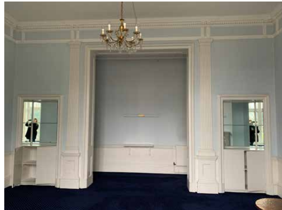
Figure 4.15 Openings in this wall, located behind the rear wall of the main entrance hall, have been infilled with modern cupboards. These features are considered to detract from the interest of the room
