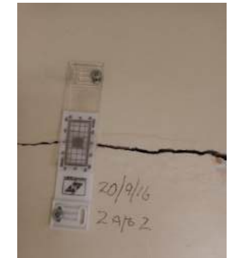
Photo 2 Movement gauge showing minimal further movement to one of the solid walls at level 3 Kneller Hall main house (west wing)
