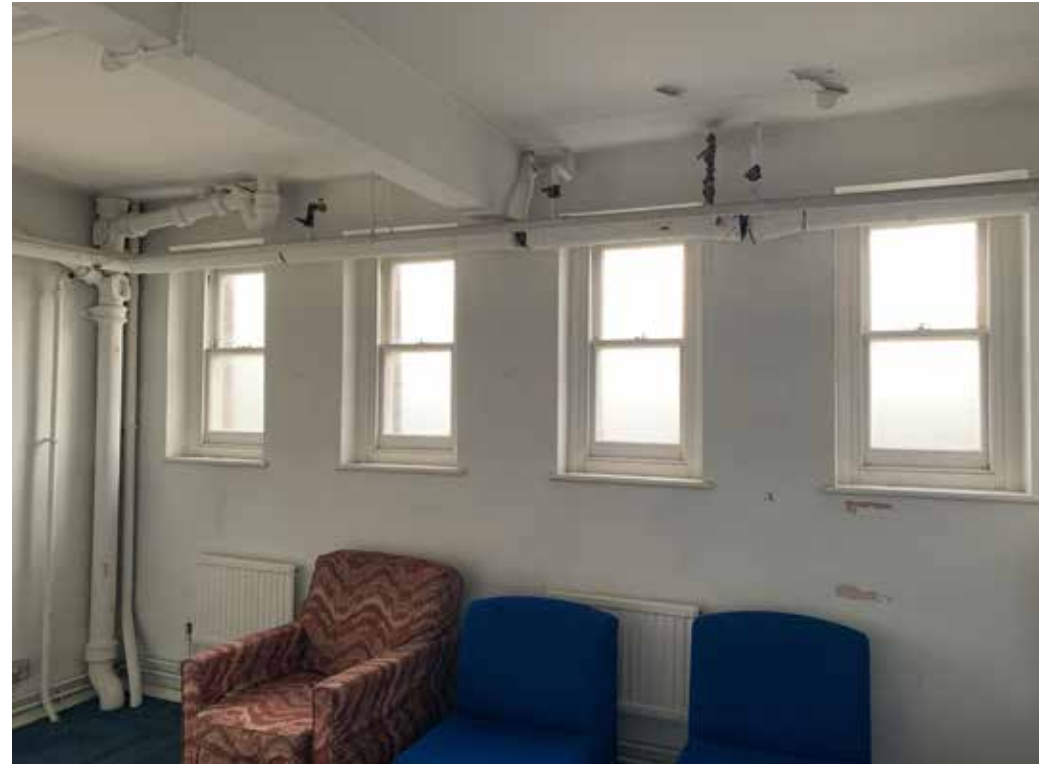
Figure 4.25 The presence of modern MEP equipment is typical within rooms located in the west wing
