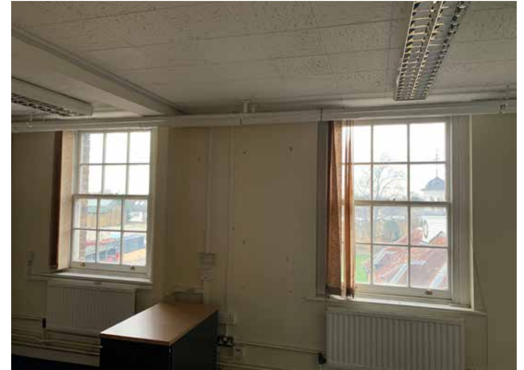
Figure 4.27 A typical modern dropped ceiling located within the west wing conceals the tops of historic windows and negatively alters the historic volume of the space
