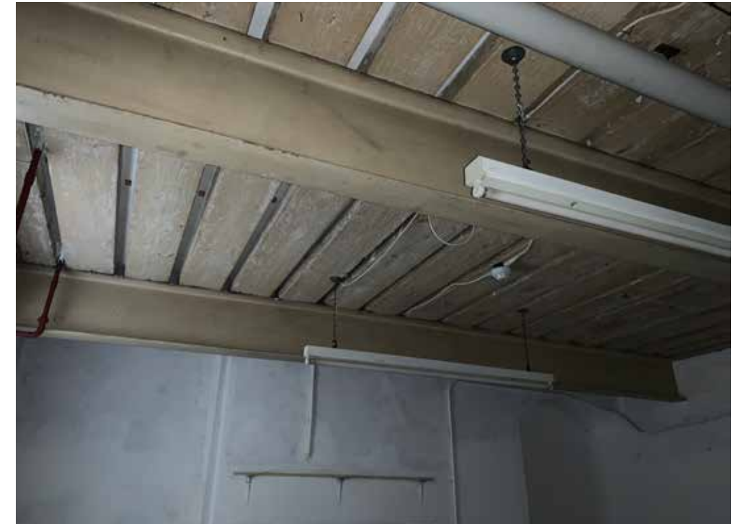
Figure 4.7 Modern ceiling beams and joists have been introduced in many rooms within the basement and replace historic features
