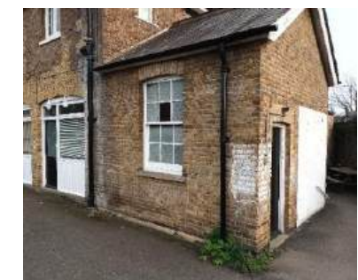
Photo 4 Failed Brick Arch above sash window at the rear storage room in the Guards House
