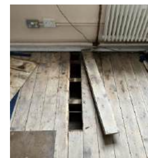
Photo 3 Opening up works showing existing floor joists at the first floor in the Guards House
