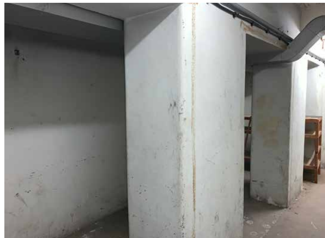
Figure 4.6 Early nineteenth-century supportive columns in the basement. Modern MEP equipment has been inappropriately fitted here.
