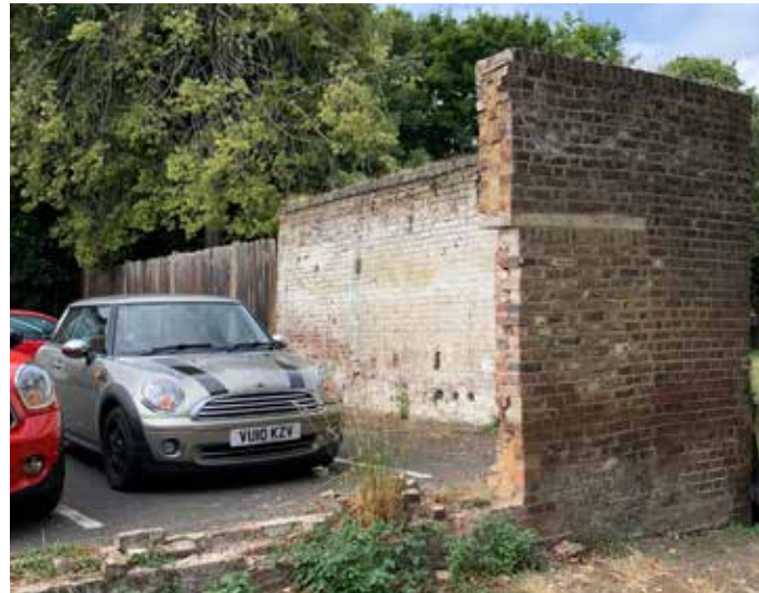
Figure 3.49 Photograph of the surviving section of garden wall. The wall is in a state of disrepair and is structurally unstable
