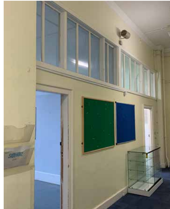
Figure 4.9 Detractive modern partition walls have been installed west of the main entrance hall. They comprise a plain design and have subdivided an historic classroom to create multiple rooms and a corridor
