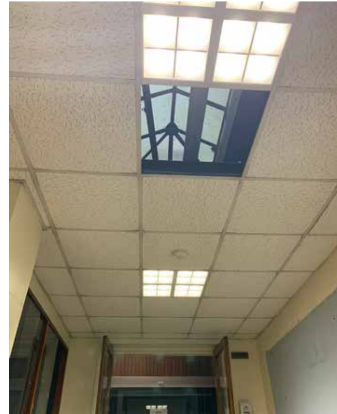
Figure 4.10 A modern dropped ceiling has been installed in the west-entrance corridor. It conceals the nineteenth-century skylight feature
