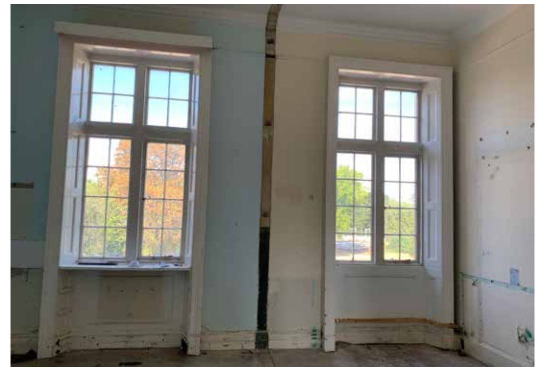
Figure 4.24 A detractive, modern partition has been removed as part of consented enabling works. This exemplifies how the removal of such partitions can reinstate the historic volume of spaces and enhance their significance
