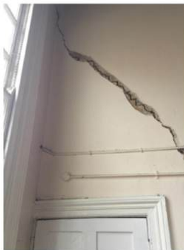
Figure 1: Cracking to Internal Masonry Wall
