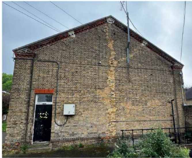
Figure 1: Cracking to West Gable Masonry Wall. Note previous brick repairs
