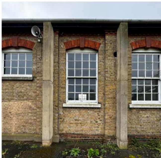
Figure 2: Cracking to North Elevation Masonry Wall above and Below Window
