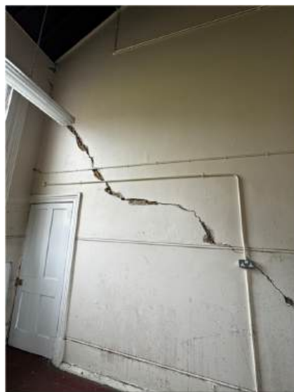
Figure 3: Cracking to Internal Masonry Wall
