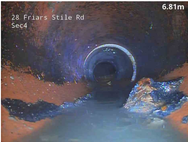
7, 00:02:12, 6.90 m Attached deposits, encrustation from 3 o'clock to 6 o'clock, 10% cross-sectional area loss
