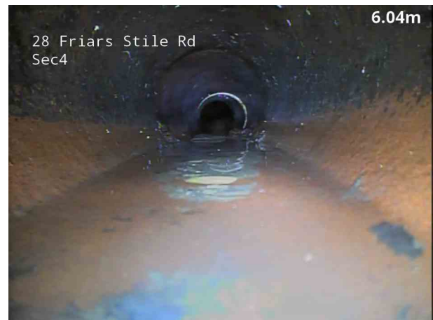
6, 00:01:35, 6.00 m Attached deposits, encrustation from 4 o'clock to 8 o'clock, 15% cross-sectional area loss, finish
