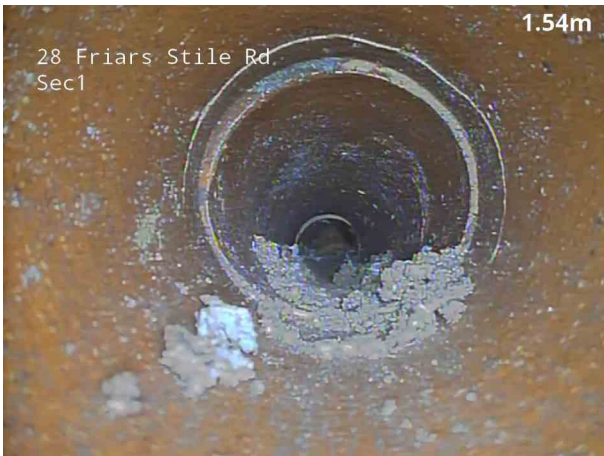
3, 00:00:52, 1.70 m Fracture, circumferential at joint from 9 o'clock to 5 o'clock
