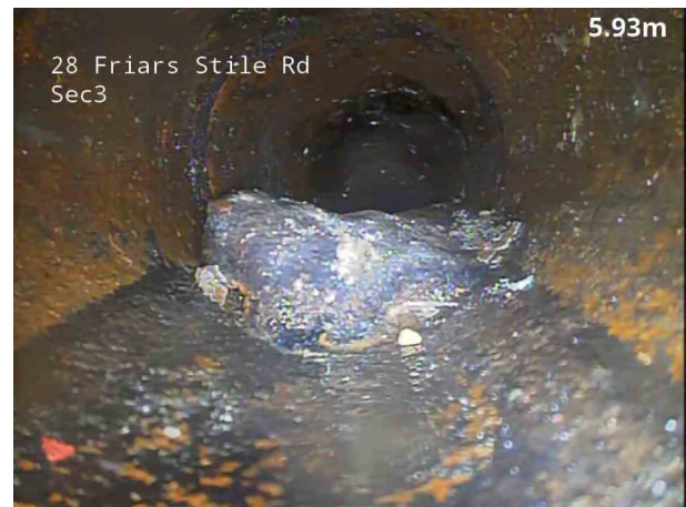
6, 00:00:40, 6.10 m Attached deposits, encrustation at joint from 4 o'clock to 8 o'clock, 30% cross-sectional area loss
