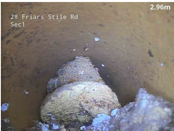
5, 00:00:27, 3.00 m Settled deposits, coarse, 70% cross-sectional area loss, change
