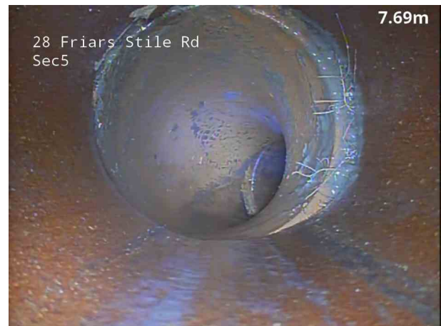
6, 00:00:13, 7.90 m Roots, fine at joint
