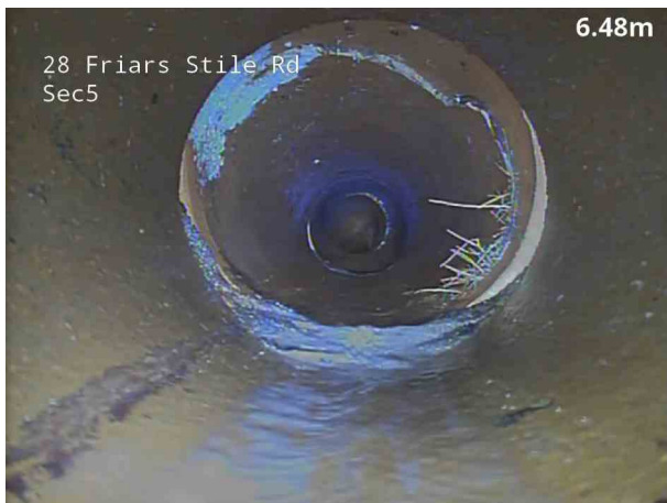
5, 00:00:23, 6.70 m Fracture, circumferential at joint from 12 o'clock to 12 o'clock
