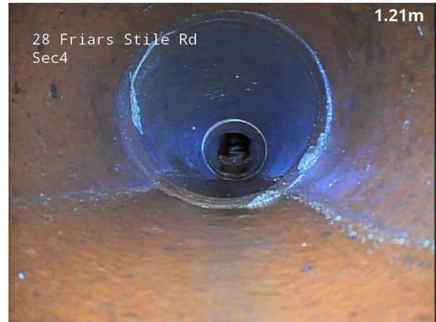
2, 00:00:29, 1.40 m Fracture, circumferential at joint from 8 o'clock to 4 o'clock
