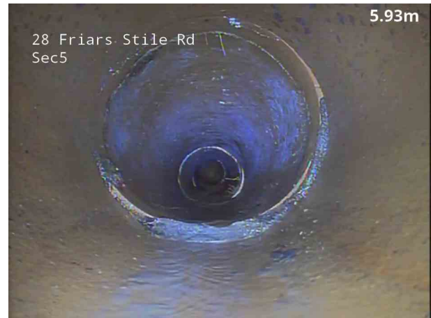
4, 00:00:28, 6.10 m Fracture, circumferential at joint from 12 o'clock to 12 o'clock
