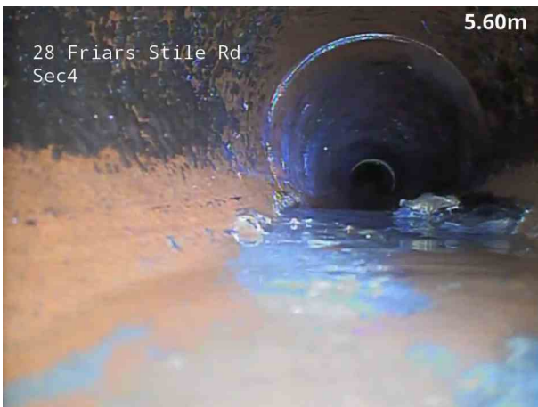
5, 00:01:23, 5.80 m Attached deposits, encrustation from 4 o'clock to 8 o'clock, 15% cross-sectional area loss, change
