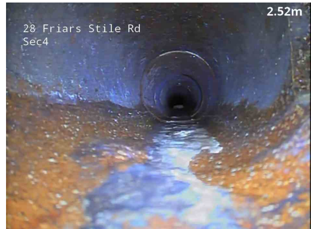
4, 00:00:47, 2.50 m Attached deposits, encrustation from 5 o'clock to 7 o'clock, 5% cross-sectional area loss, start
