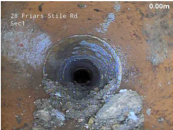
1, 00:01:12, 0.10 m Settled deposits, coarse, 20% cross-sectional area loss, start
