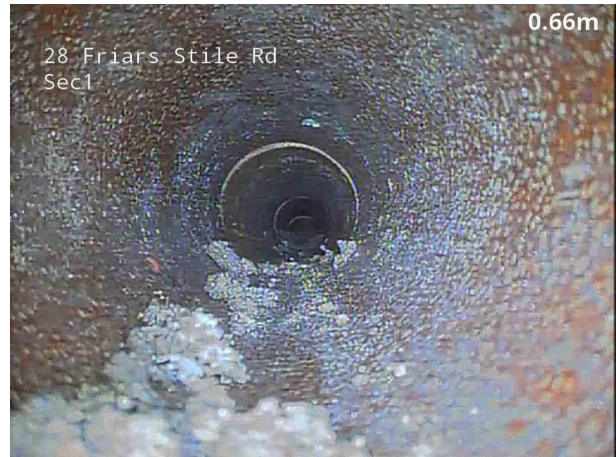
2, 00:01:01, 0.70 m Settled deposits, coarse, 10% cross-sectional area loss, change
