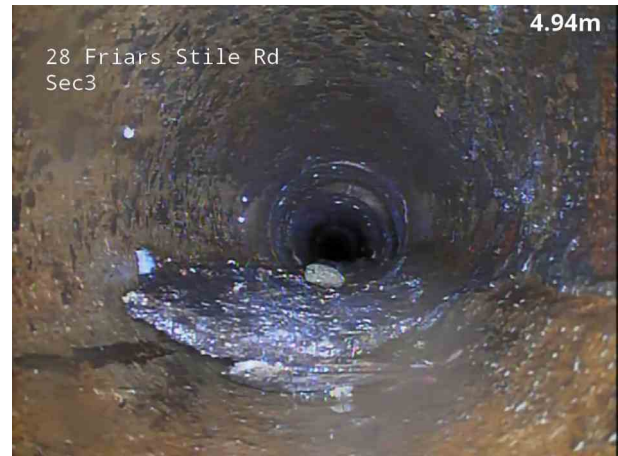
4, 00:00:56, 5.10 m Attached deposits, encrustation from 4 o'clock to 8 o'clock, 20% cross-sectional area loss
