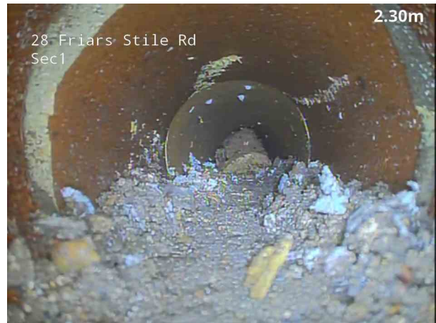
4, 00:00:40, 2.40 m Settled deposits, coarse, 40% cross-sectional area loss, change
