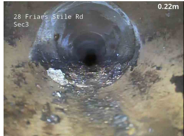
2, 00:01:30, 0.30 m Attached deposits, encrustation at joint from 4 o'clock to 8 o'clock, 15% cross-sectional area loss
