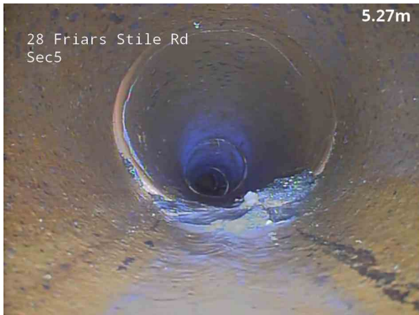
3, 00:00:32, 5.50 m Fracture, circumferential at joint from 7 o'clock to 3 o'clock
