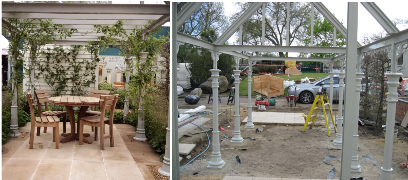
Example of the pergola structure and columns. Example of the canopy structure before glass roof installed. The canopy has glass to the roof and gable ends but is open around the columns.
