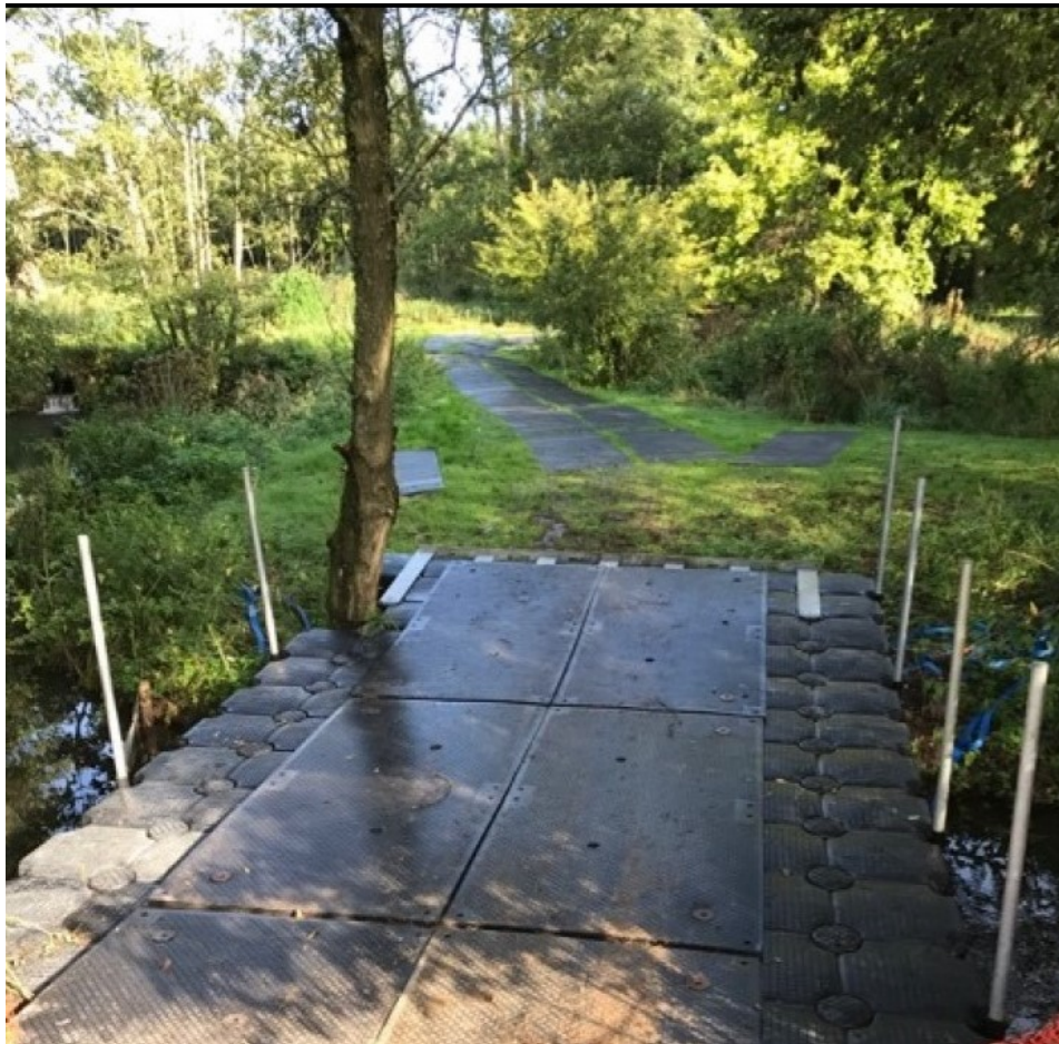
Fig. 1 Ground Guards – MultiMatts Euro Trak is ideal for the ground protection required here.
