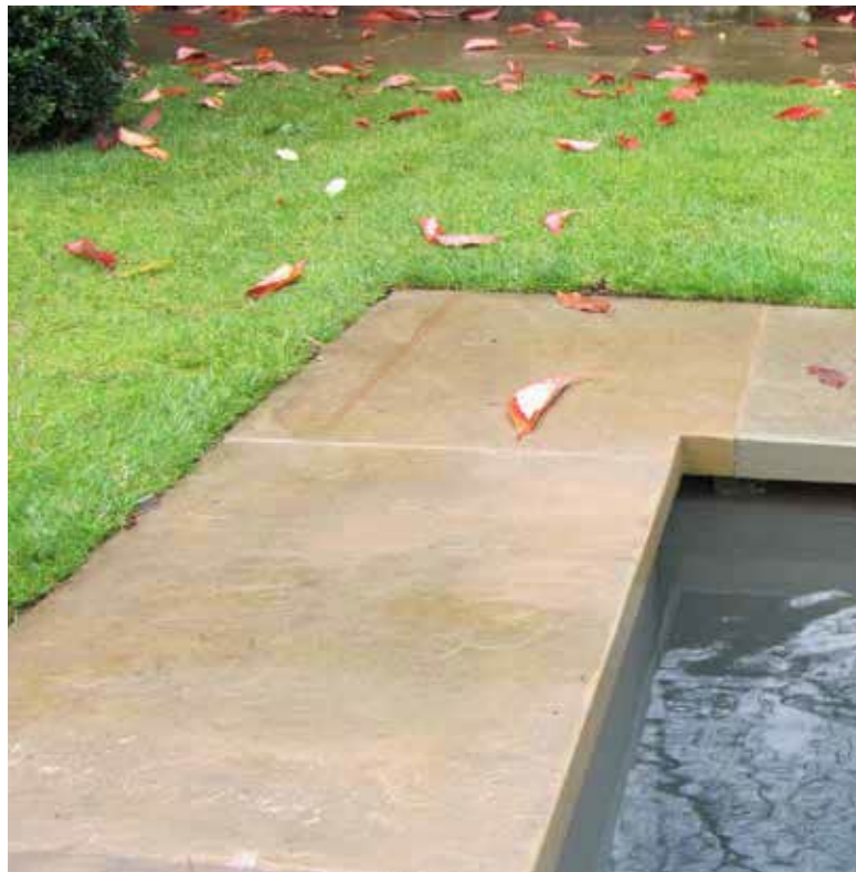
Reclaimed York stone pool coping
