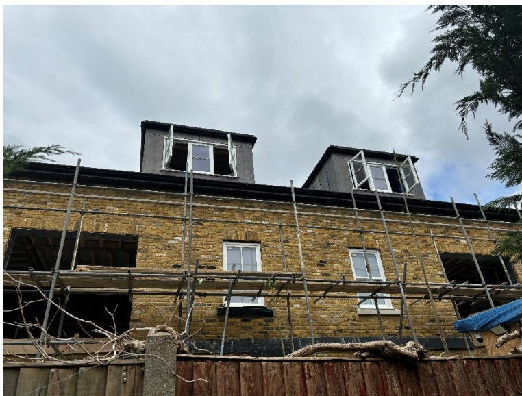
Image 10 - Rear dormers significantly overlooking neighbour gardens
