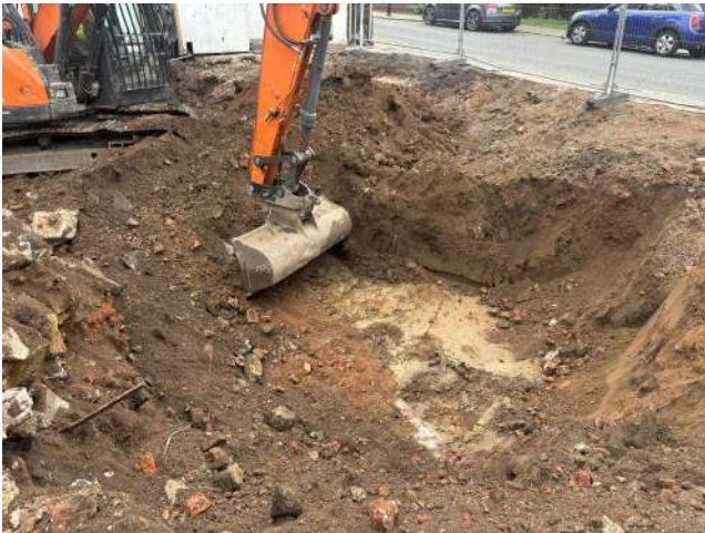
Photo Five: Removal of temporary backfill / exposing clay layer, prior to soil sampling.
