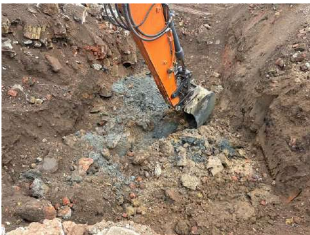
Photo Seven: Excavating through the clay layer, in order to facilitate soil sampling from the underlying sand/gravel layer.
