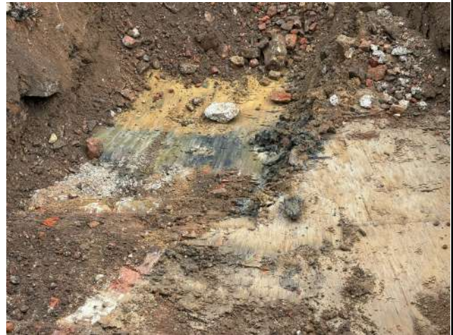
Photo Six: The surface of the upper clay layer (present directly beneath the former tank farm), with some limited areas of hydrocarbon staining.
