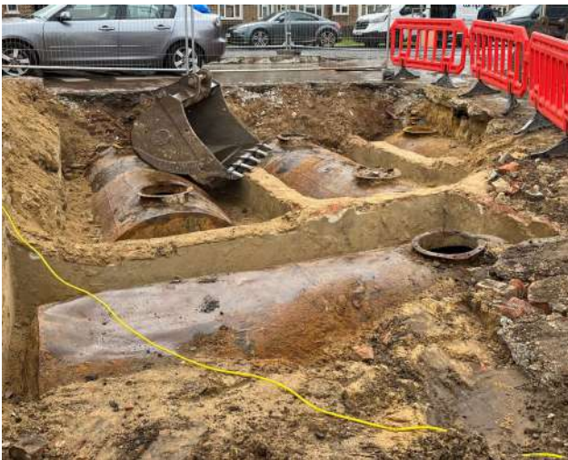
Photo One: Abandoned fuel tanks, prior to removal.
