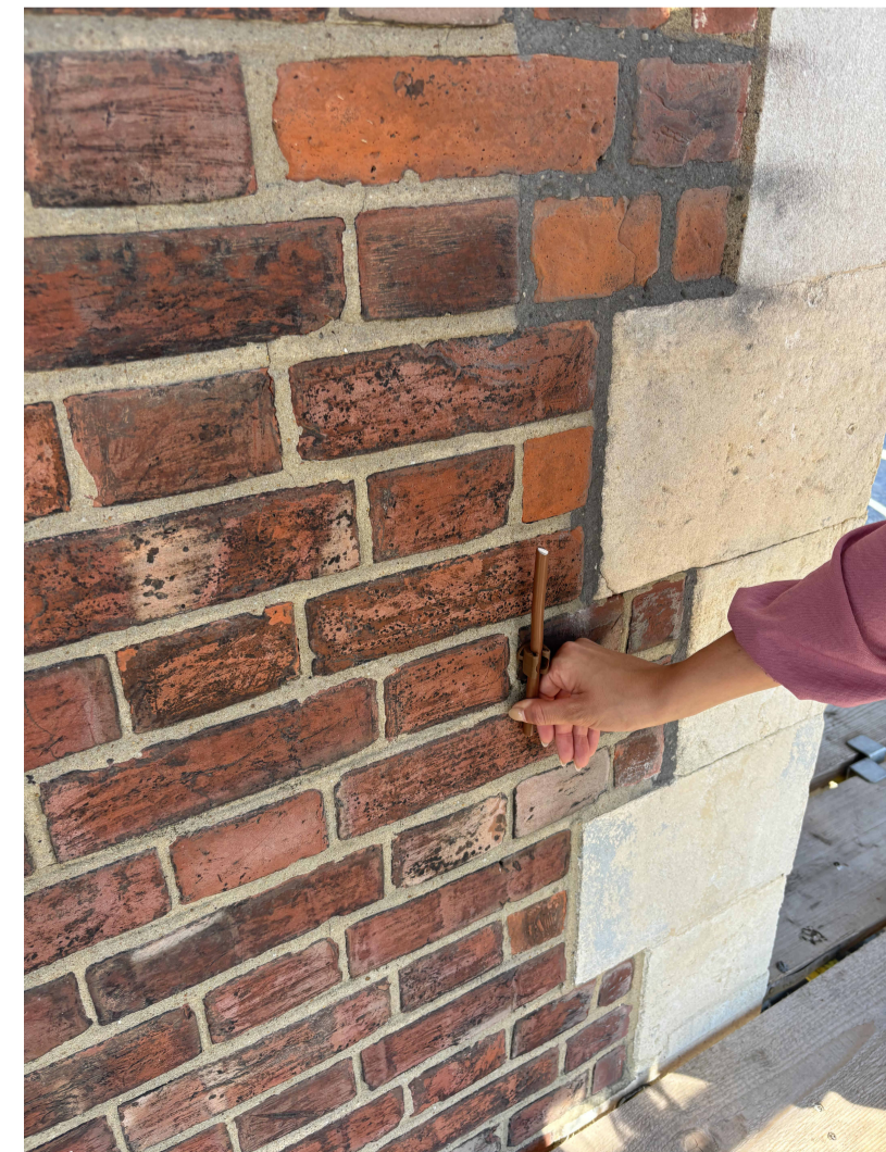
Image 1 Thin copper Lightening Protection tubes dropped down on elevations as per locations on drawing above
