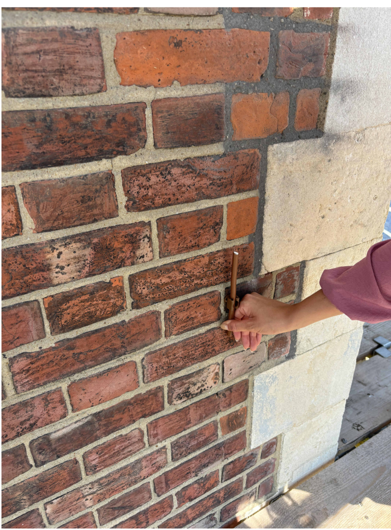
Image 1 Thin copper Lightning Protection tubes dropped down on elevations as per locations on drawing above
