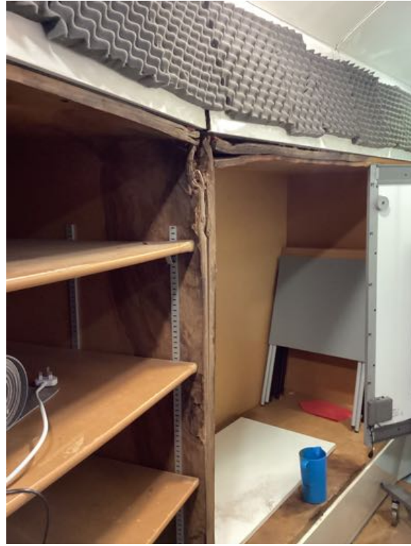
Water damaged shelving at the rear of the Ingenium Pod
