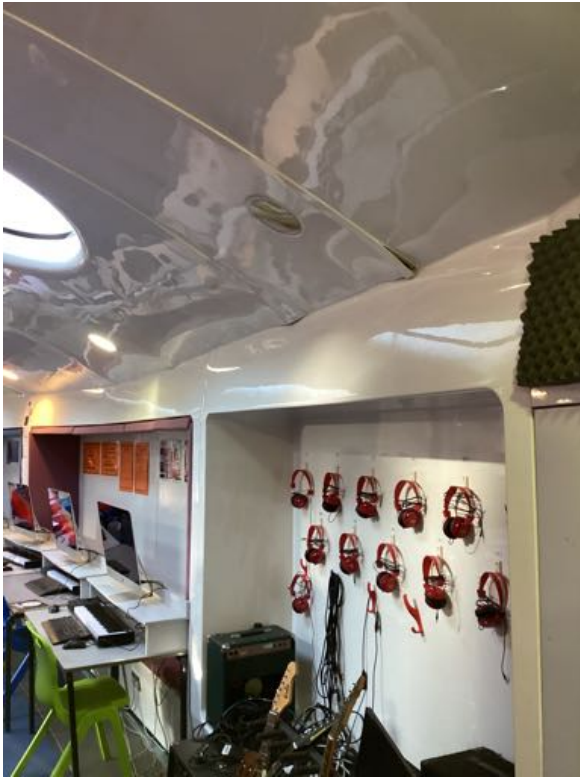
Ill-fitting internal wall lining panels due to overall distortion of the shell
