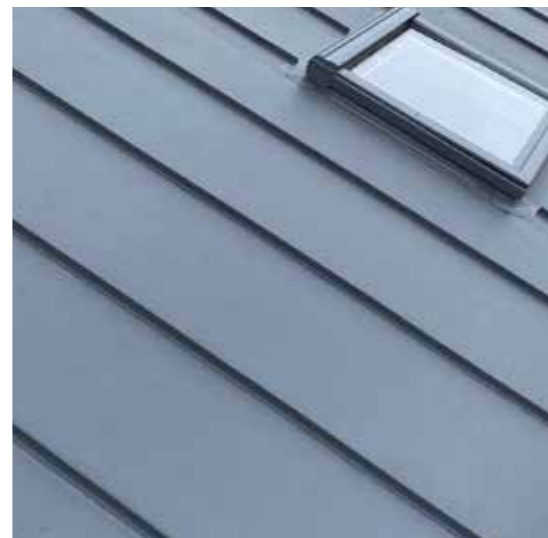
6. Single ply waterproof membrane Single ply roofing membrane with the appearance of a standing seam roof.
