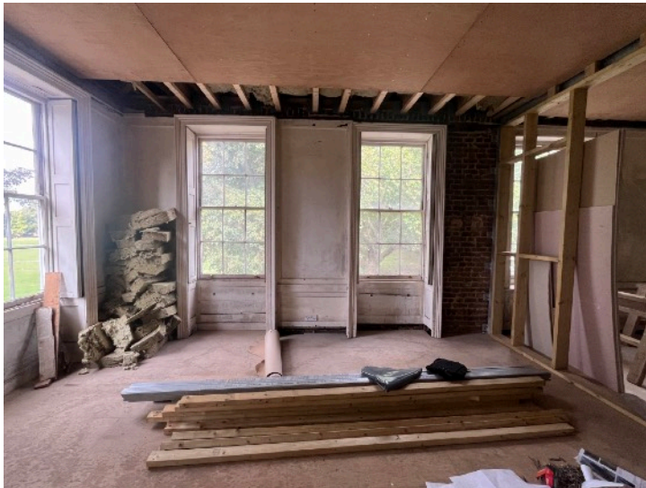
Figure 8: Room F2 showing the original panelling and modern floor joists with original timbers between
