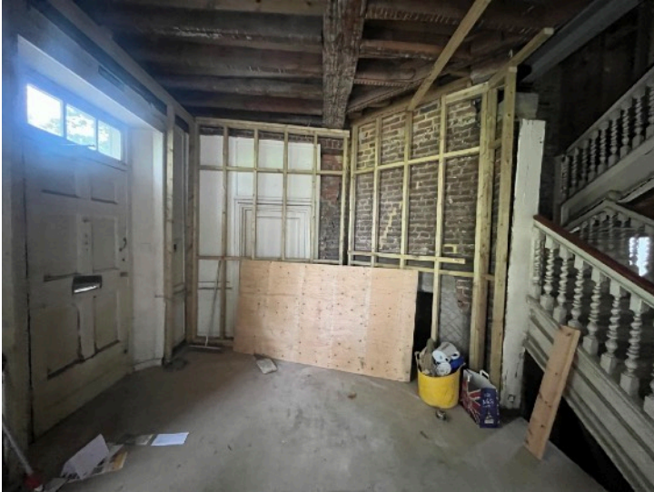
Figure 10: Room G3, entrance hall looking towards the redundant doorways once connecting to No. 31 and the stair to the right
