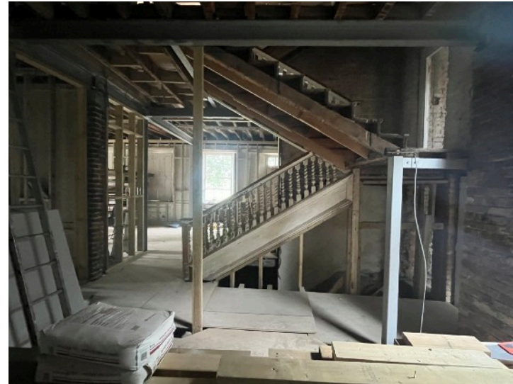
Figure 7: Photo from Room G4 across stairwell to main entrance door showing the installed steel frame
