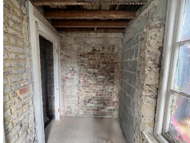
Figure 11: Room S5 to Second Floor Rear Extension looking towards the party wall to no. 32 and the various blocked up doorways
