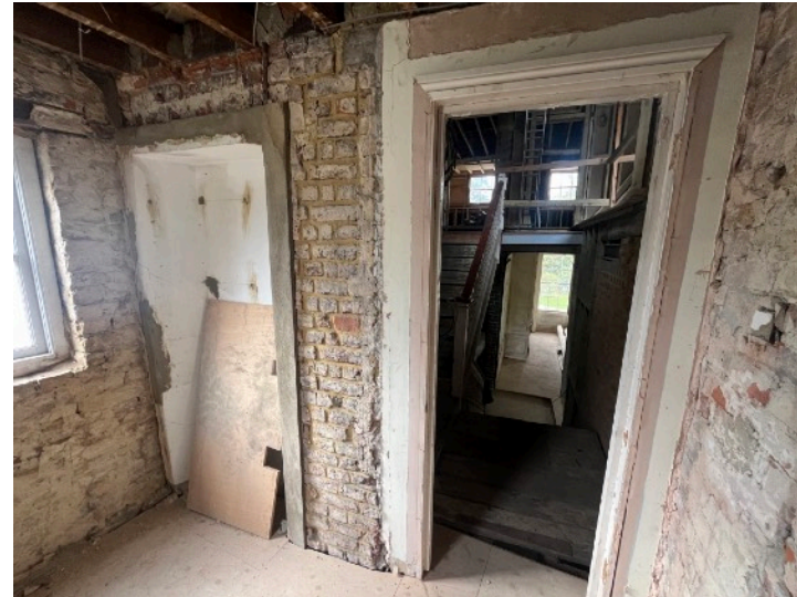
Figure 13: Room S5 to Second Floor Rear Extension looking towards the stairwell with blocked up doorway to the left
