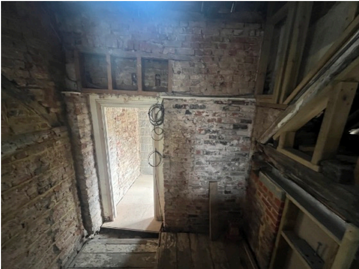
Figure 12: Standing on Second floor landing looking down to the half landing where there may have been a window
