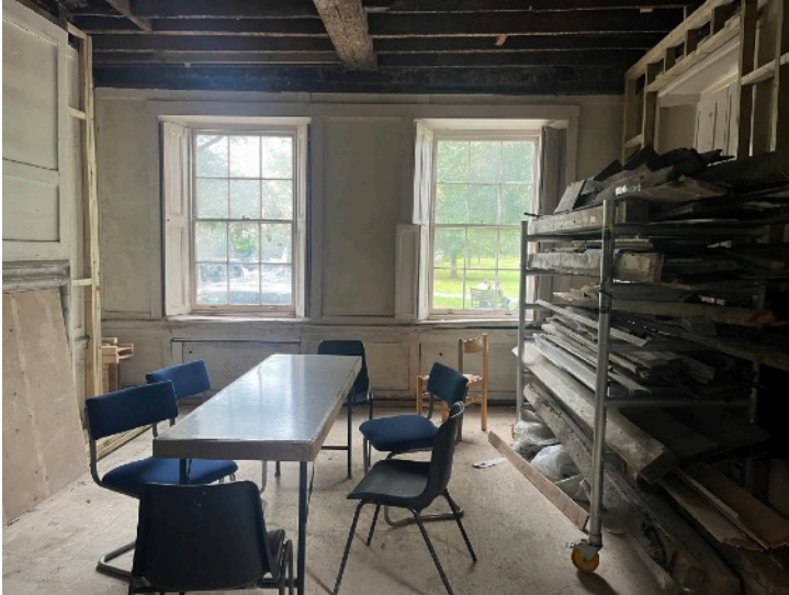
Figure 6: Room G2 with original panelling to walls and some stud work over. Also labelled and stored materials from removed panels to a rack
