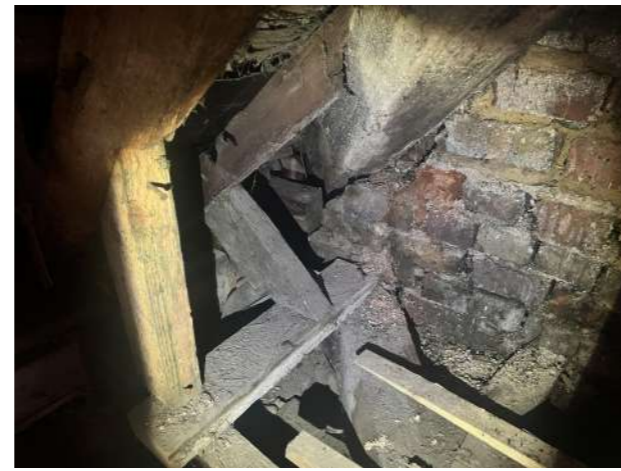
End of hip extending at corner, connection to end of diagonal floor beam / not seen.
