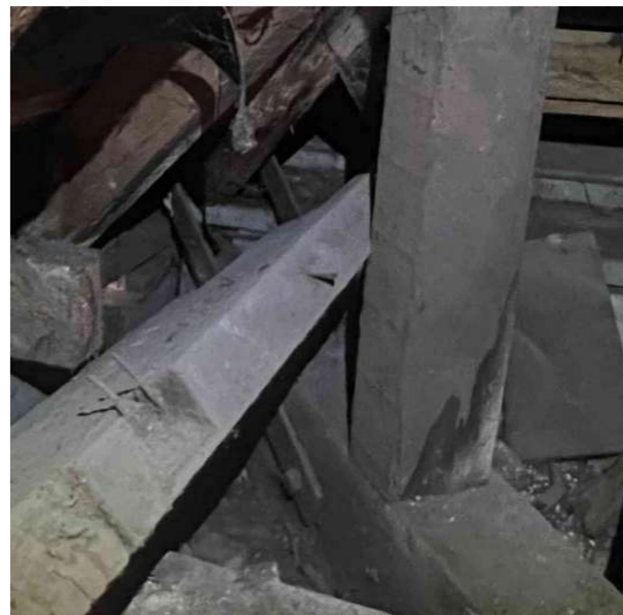
End of hip extending at corner, metal strap connection to end of diagonal floor beam holds the hip down and resists outwards thrust.
