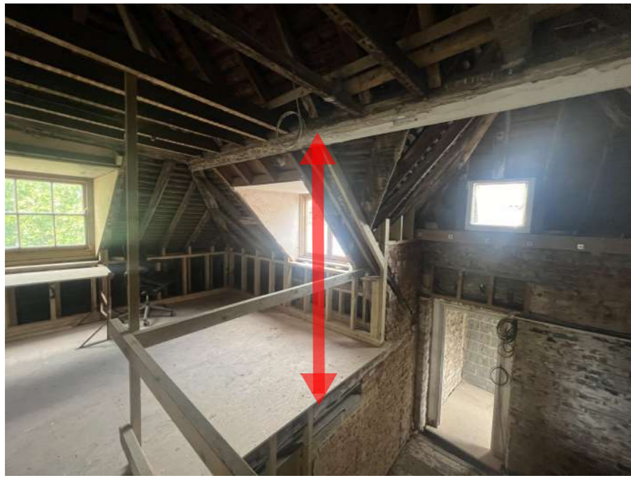
The purlin's span is too great for its size.
