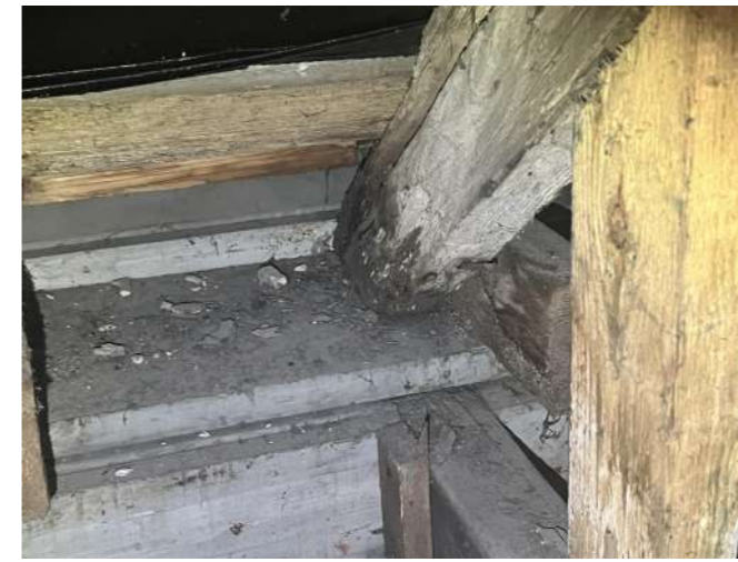
Interior view of cornice. Note grey colour, suggests replaced. Due to outward movement? Also Note decayed Rafter foot.
