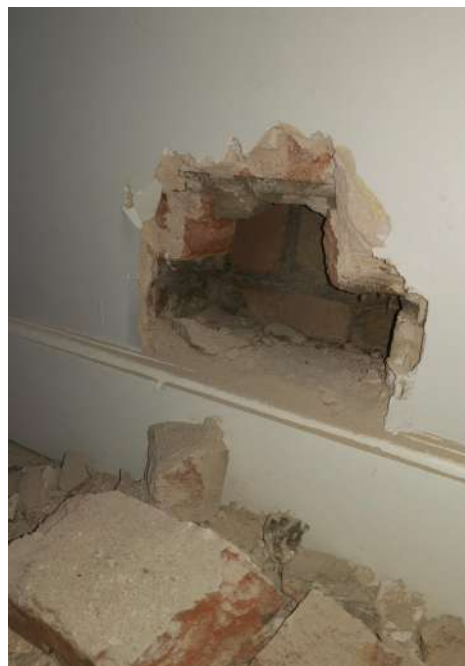
Fire box blocked up
