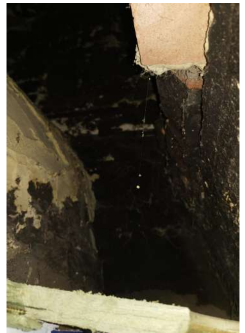
Damper with smoke chamber above
