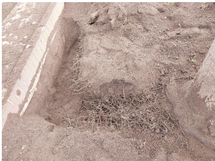
View of trial pits on the north side of the stem with visibly more roots but still no roots close to the hard standing
