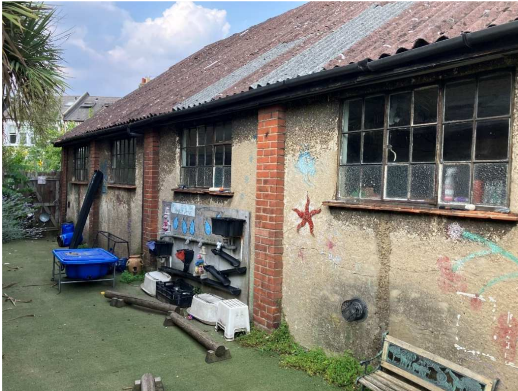
View of the Church Hall showing the asbestos roof, rendered walls and single glazed steel Crittall windows
