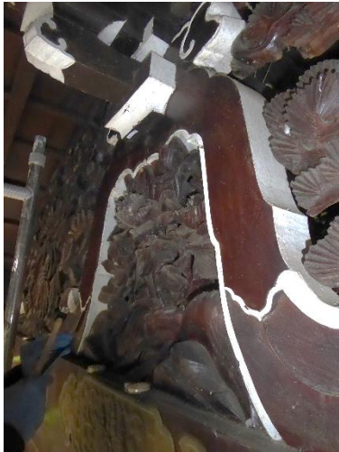
Figure 16: South elevation, decorative brace, showing the areas picked out in white paint.
