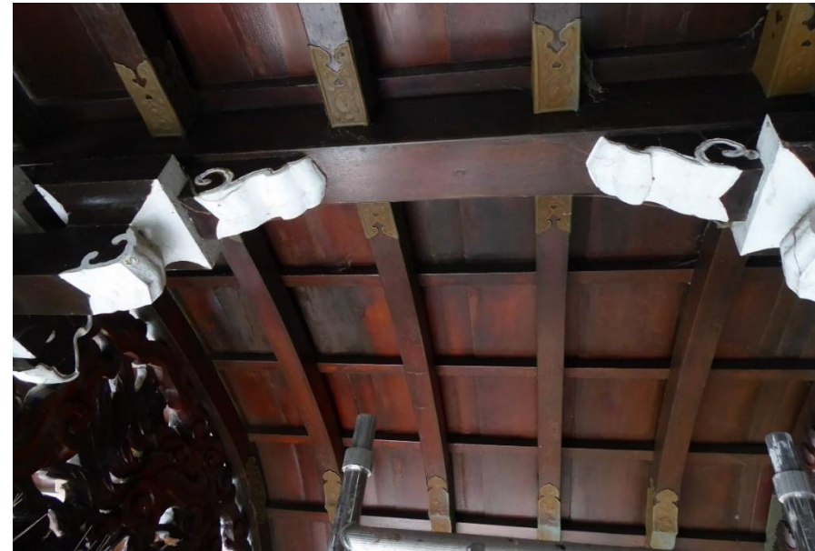
Figure 7: Image showing the ceiling timbers on the south side of the structure.
