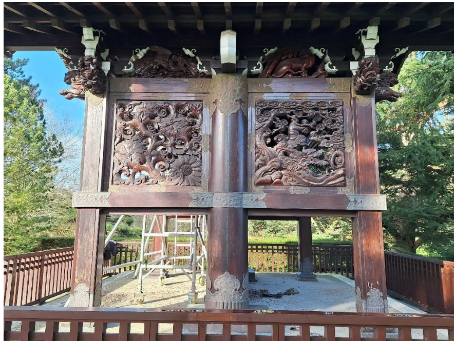
Figure 8: East elevation, showing the increased deterioration of the painted surfaces to the south (left) compared to those on the north side (right).
