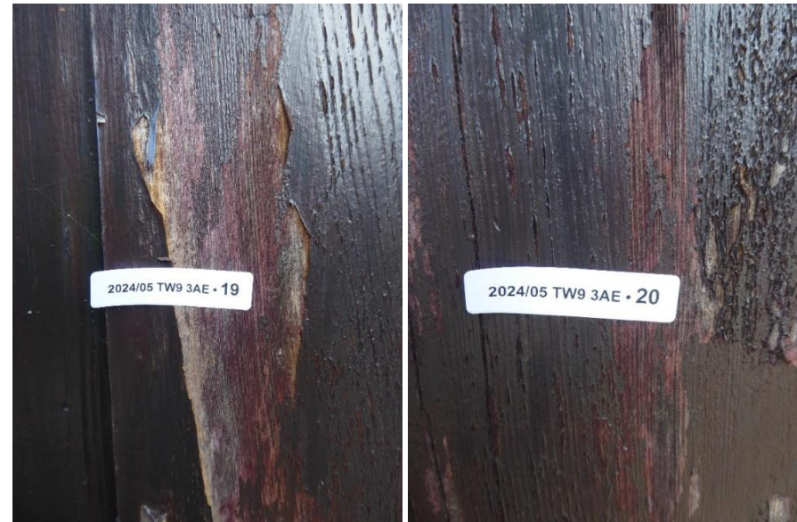
Figure 9: Images showing the red colour beneath the peeling films on the south-western post.
