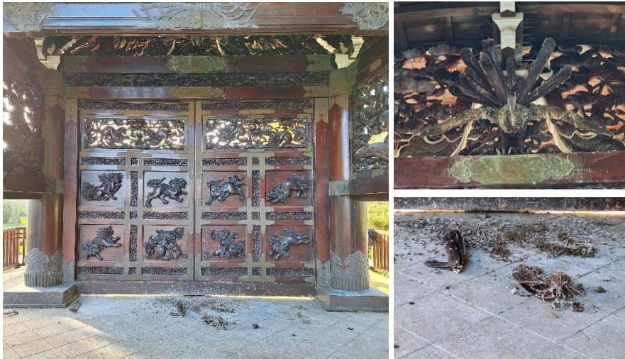
Figure 10: North elevation, showing the damaged decorative carvings and evidence of bird roosting.
