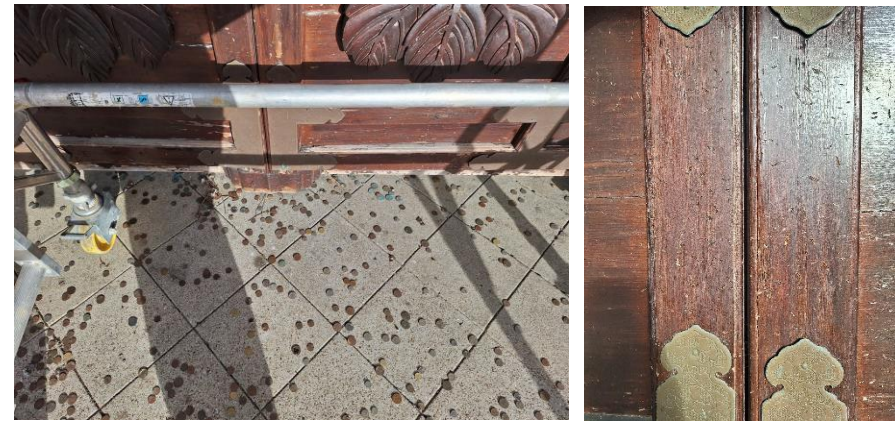
Figure 11: Image of south elevation doors, showing the damaged caused by coin offerings.
