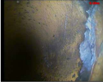
Observation [1]: Start Point: STORM WATER MAMHOLE 1
