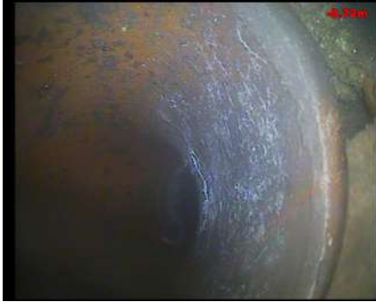
Observation [1]: Start Point: STORM WATER MANHOLE 1
