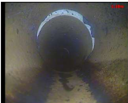
Observation [4]: MISALIGNED & OPEN JOINT
