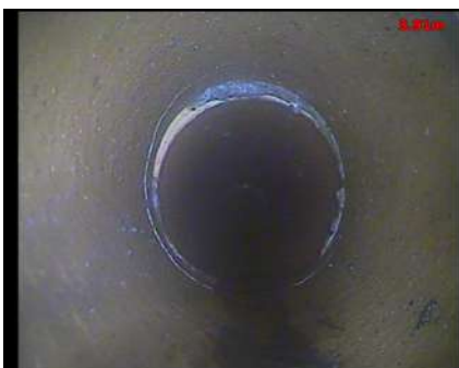
Observation [5]: CIRCUMFERENTIAL CRACK
