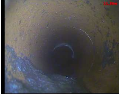
Observation [6]: CIRCUMFERENTIAL CRACK
