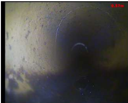
Observation [3]: CERCUMFERENTIAL CRACK
