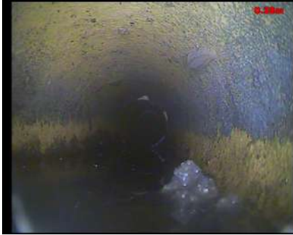
Observation [1]: Start Point: STORM WATER MANHOLE 1
