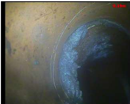
Observation [3]: CIRCUMFERENTIAL CRACK
