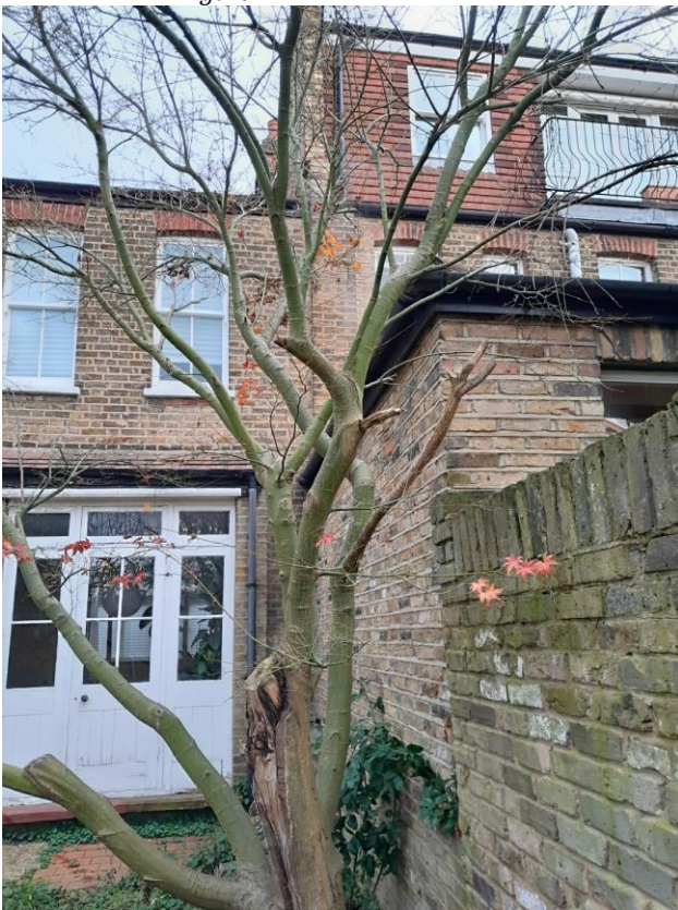
Figure 4 - T1: Encroaching onto building
