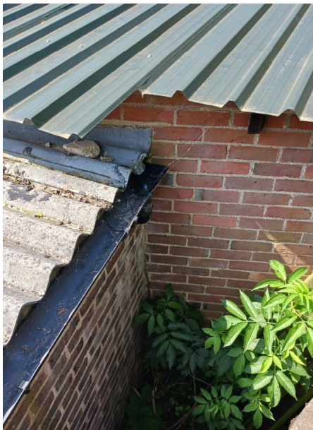
PVC Gutters and failed flashings to north elevation.
