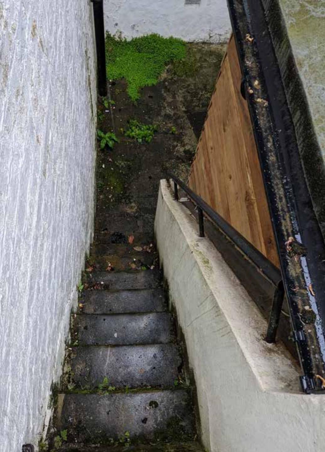
Current access down to courtyard via steep, slippery steps, proposed to be replaced with wider, shallower steps within internal enclosed courtyard
