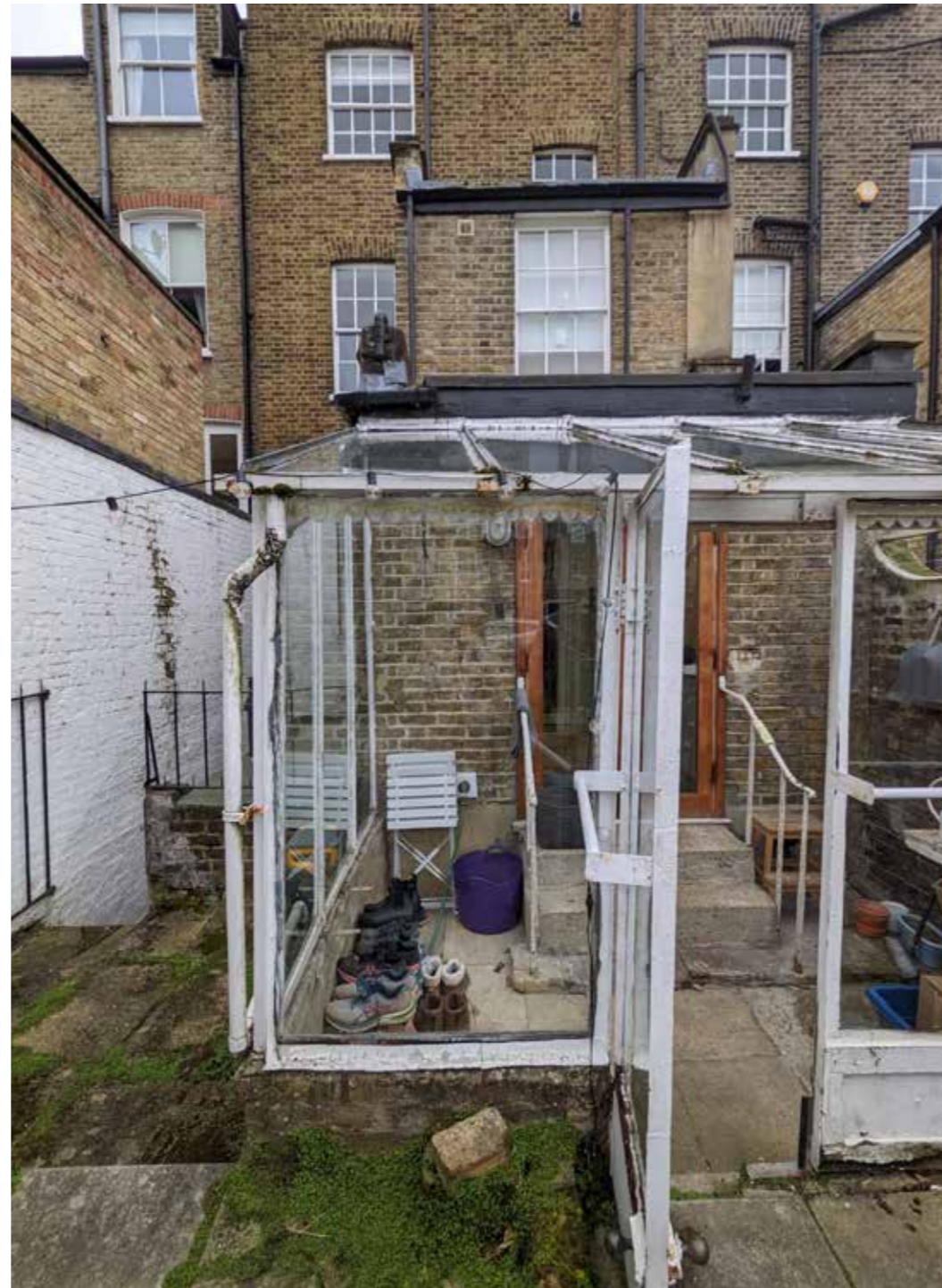
existing low quality rear extension (now removed) to be replaced with approved half width rear extension creating improved connection to rear garden
