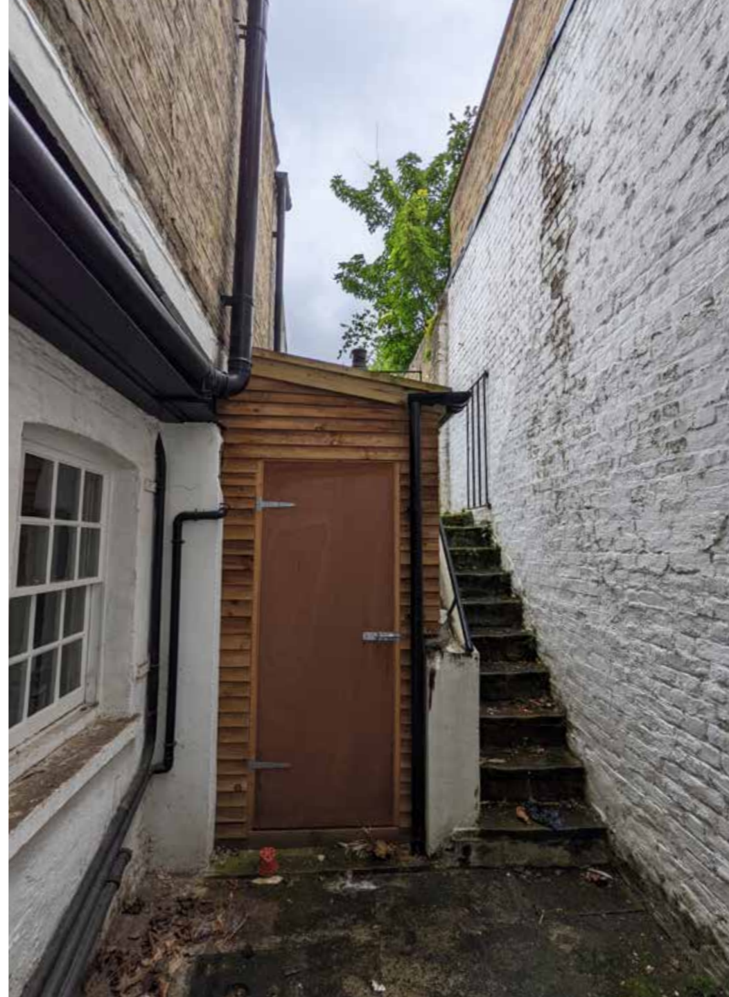
View within courtyard towards boiler shed enclosure (to be removed) with no.42 extension right of view above boundary wall
