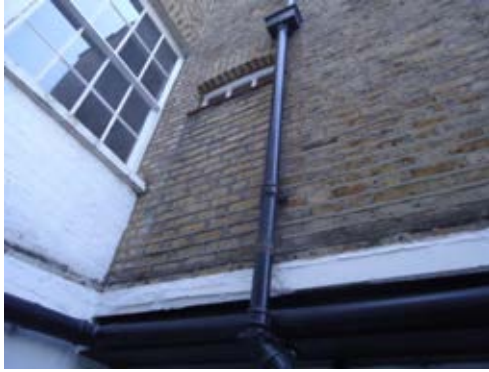
Figure 7: Overhang and filled in opening of ground floor outrigger
