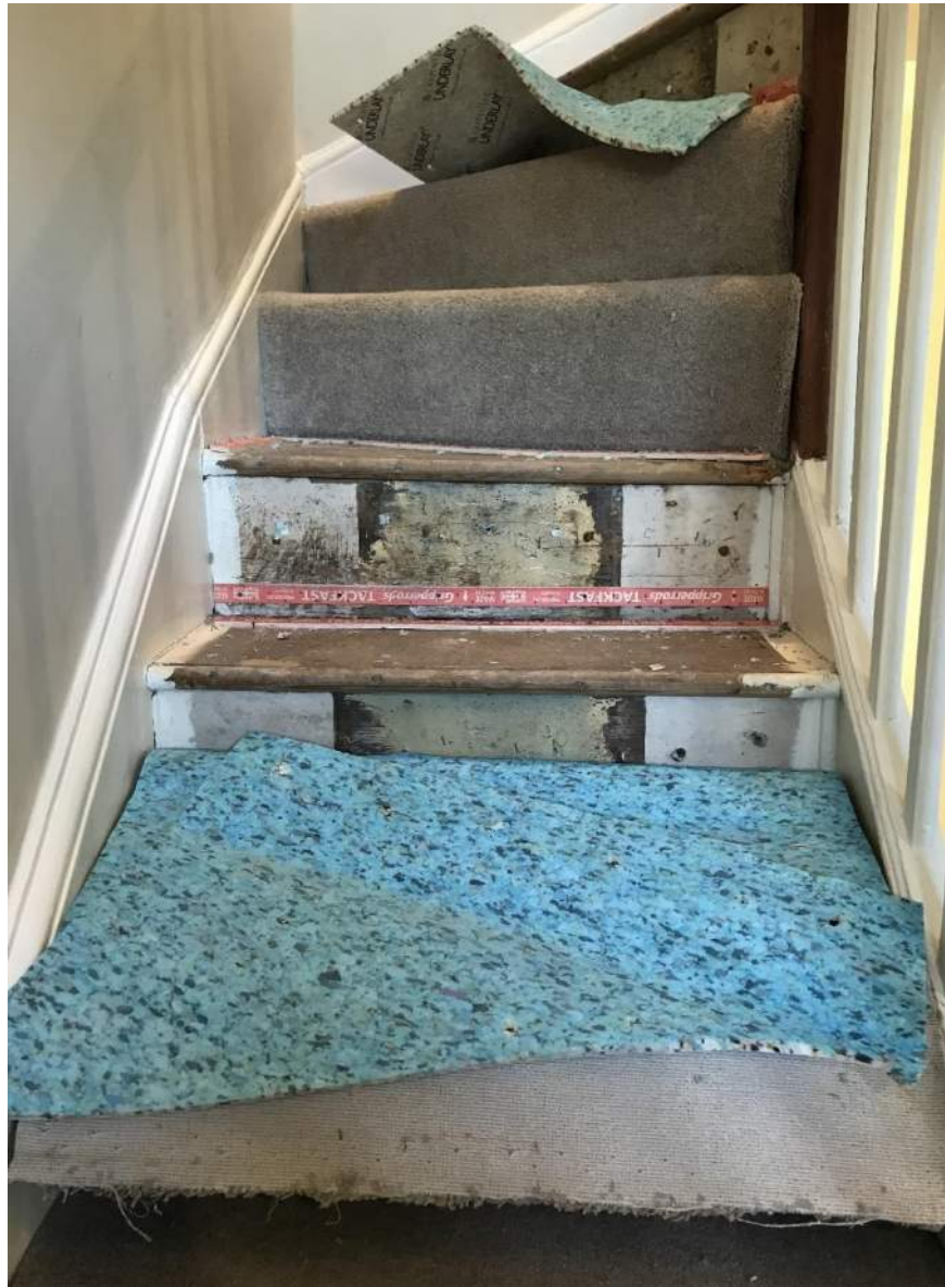
Figure 80: Carpet lifted to staircase revealing plywood treads and line of narrow runner
