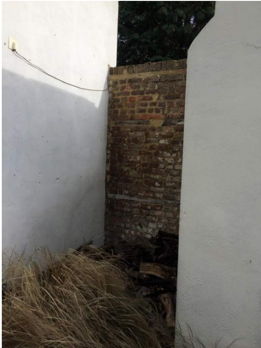
Figure 126: Section of brick-built wall, mid-20 th century, probably reusing material from the site
