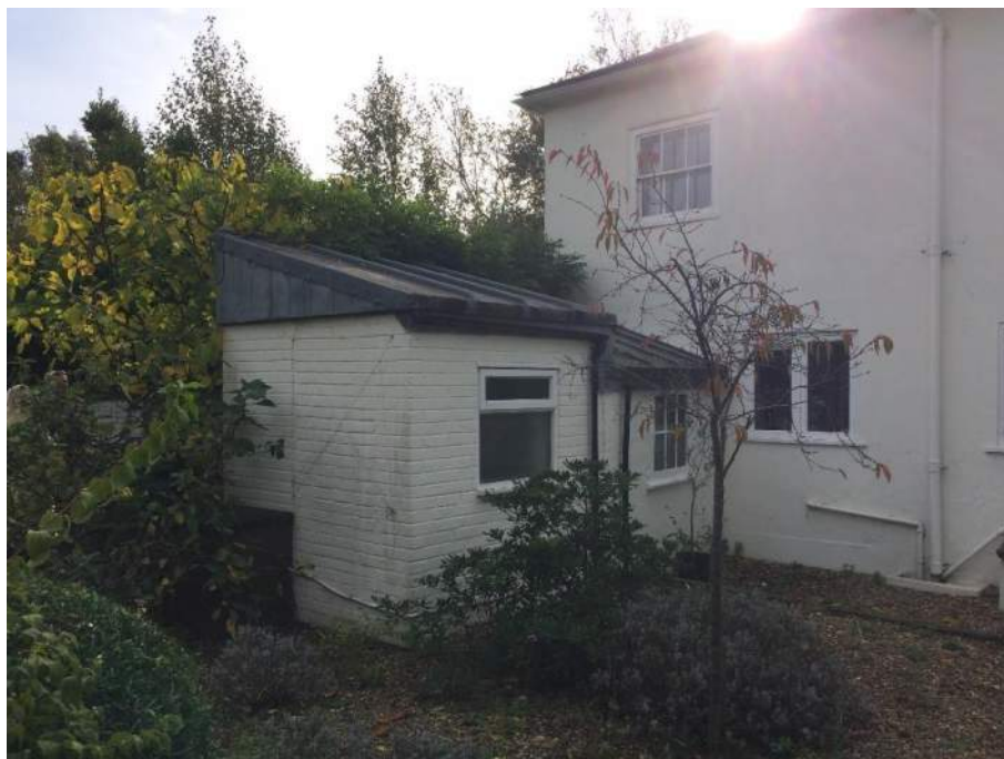
Figure 63: Extension to the north-east, first built 1911, reconfigured 1958, and rebuilt again since then
