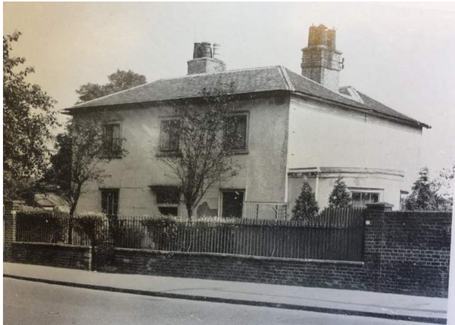
Figure 24: The Rosery, photographed for sale details in 1949; note the damaged section of stucco to the front, right of the main entrance door Surrey History Centre, SP12/18
