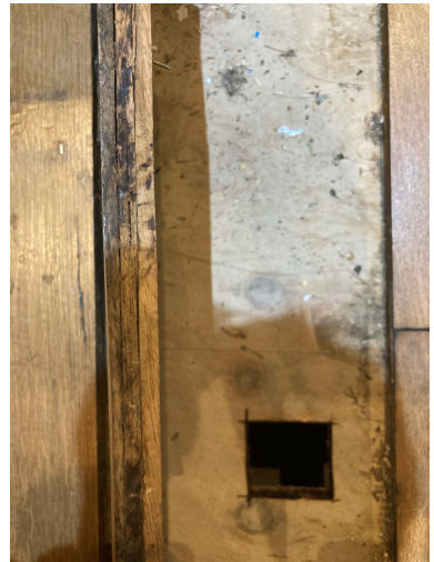
2 - Photo Close Up - Showing engineered flooring (no original flooring remains in the property). We assume existing joists are original and will be retained.
