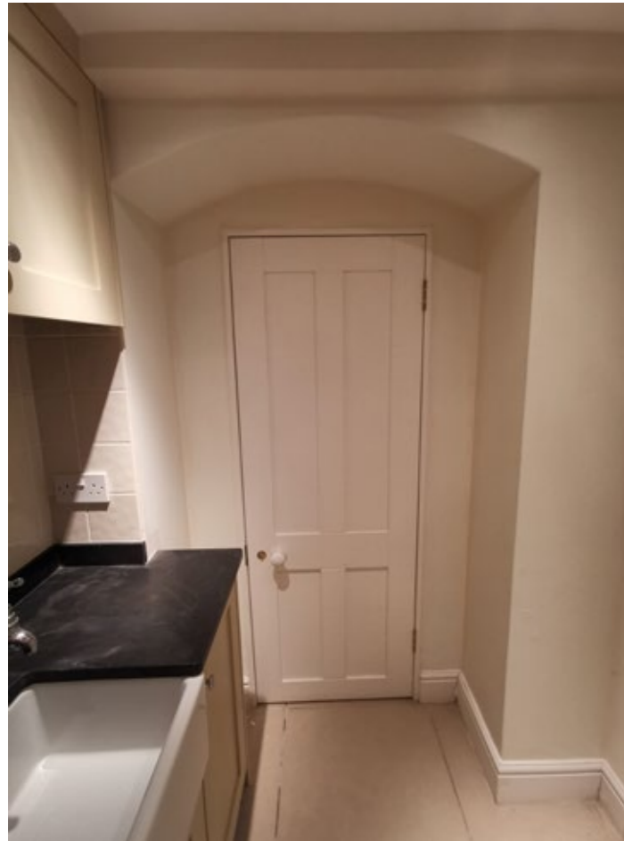
Plasterboard partition covering arch to vault under porch. Full arch to be reinstated, and partition removed
