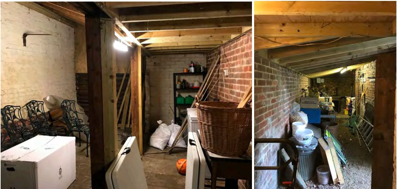
Fig.09: Internal views of existing low quality storage areas
