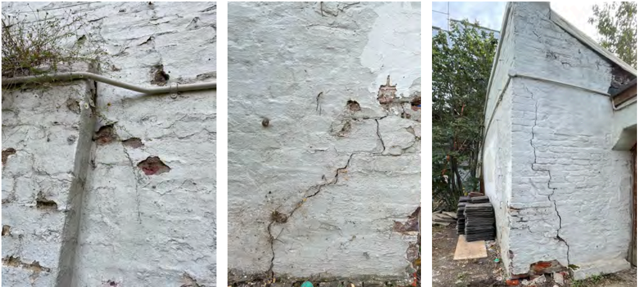
Fig.07 These images show the disrepair of the existing structure.
