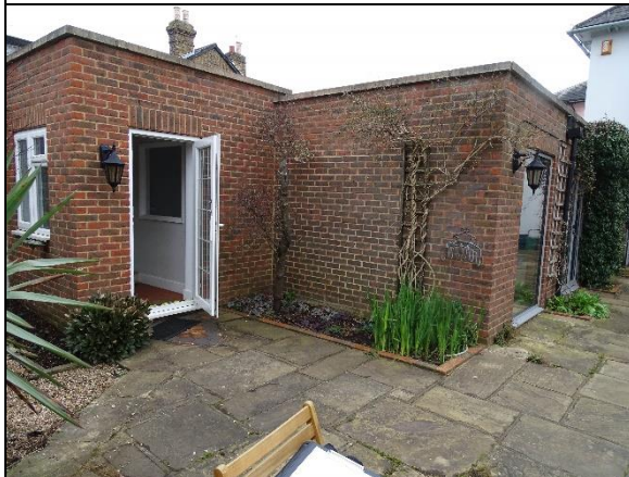
Photo 21: Sealed brick tile ridge and slate tile roof of former coach house
