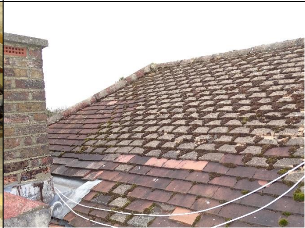
Photo 10: Rear of pitched roof (northern aspect) as viewed from external hatch to roof
