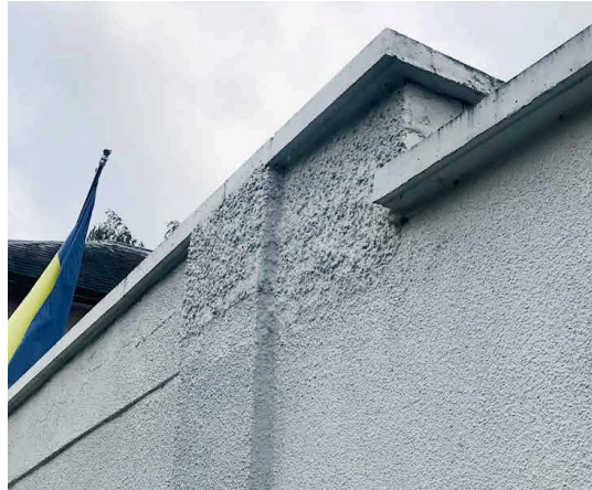
Awkward step up not aligned with pier
