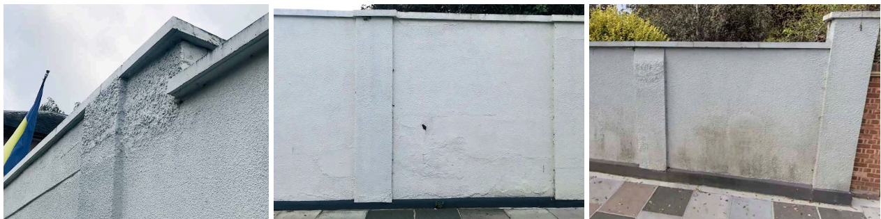
Various photographs showing examples of the condition of the rendered wall.
