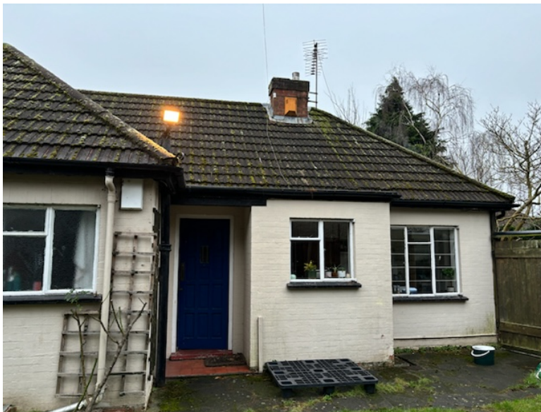
Front elevation of house showing existing flat roofed extension which it is proposed to remove
