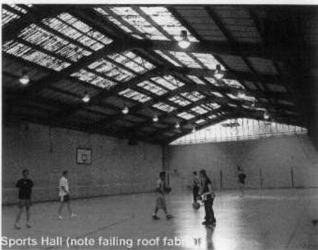
Sports Hall (note failing roof fabric)
