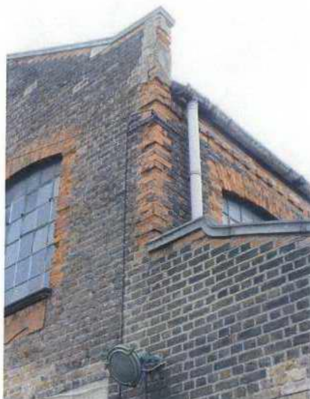
BUILDING 3 - CONDITION OF SOFT RED BRICKWORK
