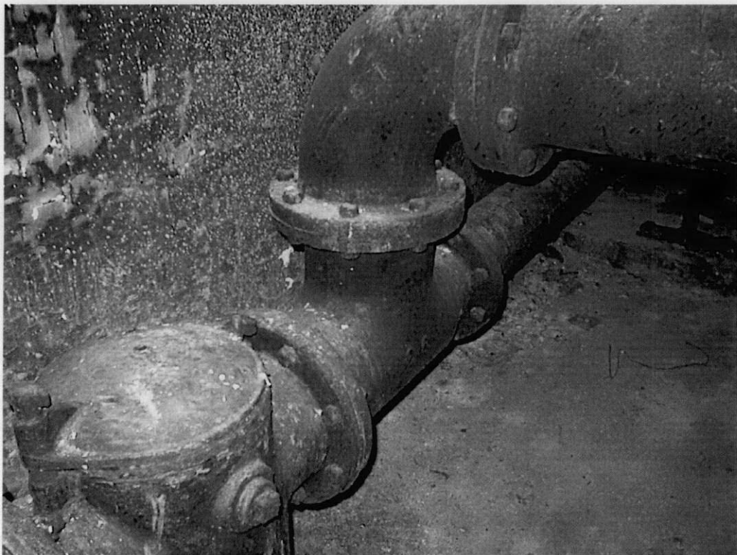
Plate 14 - Changing Block - pipework in northeast plant room on lower level
