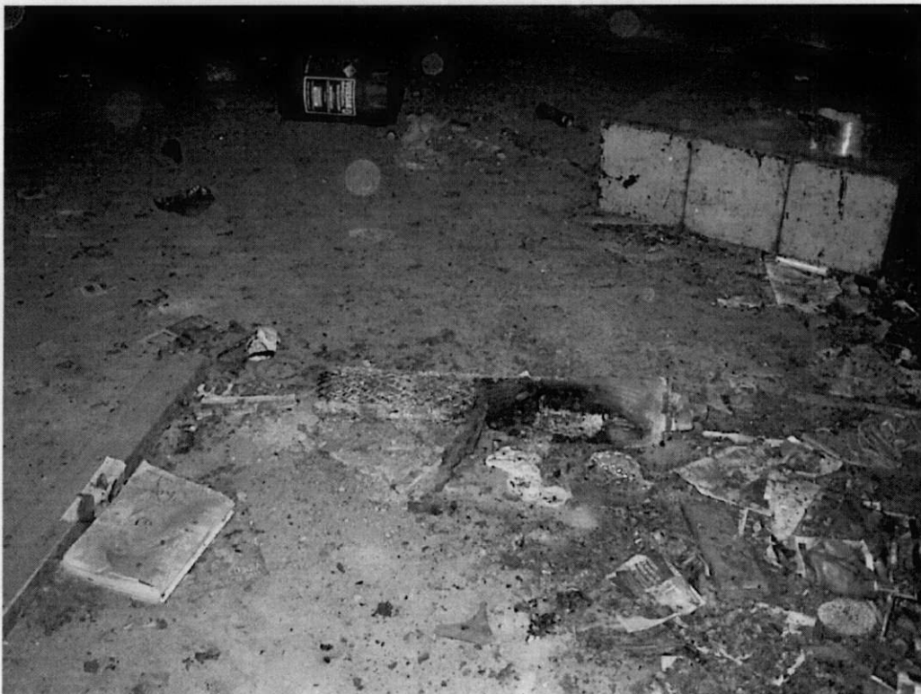
Plate 8 - Changing Blocks - redundant pipe unit in southwest plant room on lower level
