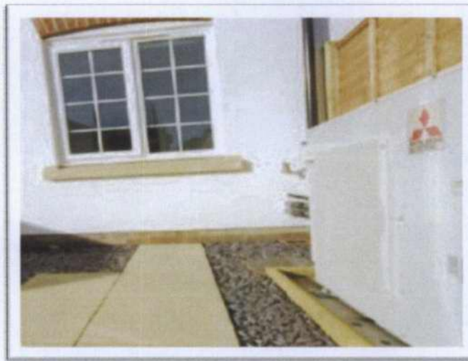
Figure 1 – External ASHP heat exchanger unit
