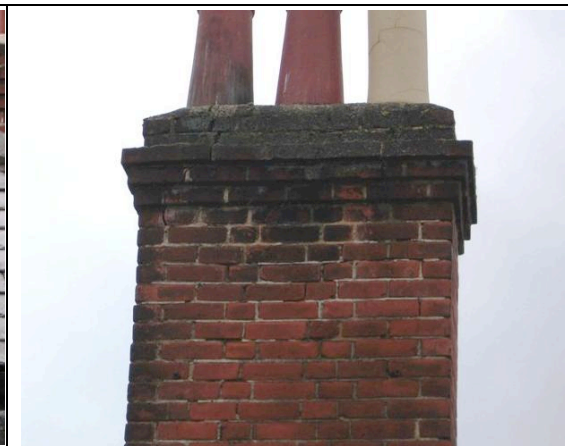
Fig. 45: Chimneystack to southeast with damaged capping and loss of mortar
