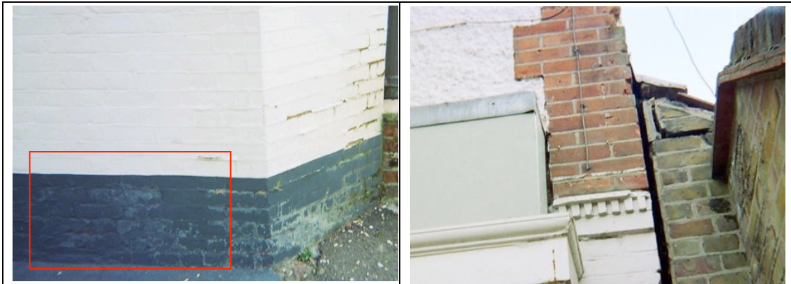
Fig. 46: Spalled brickwork at ground level
