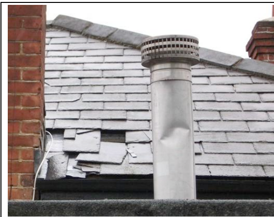
Fig. 44: Section of roof to south showing slipped and broken slates
