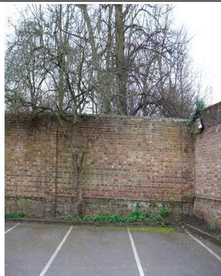
Fig. 9: A section of the wall from the car park with the neighbours later wall abutting
