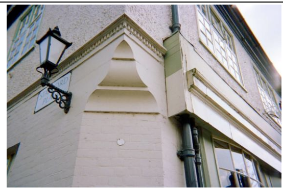
Fig. 24: Detail of section of denticulated stringcourse. Note where cornice has been truncated to allow for later fascia
