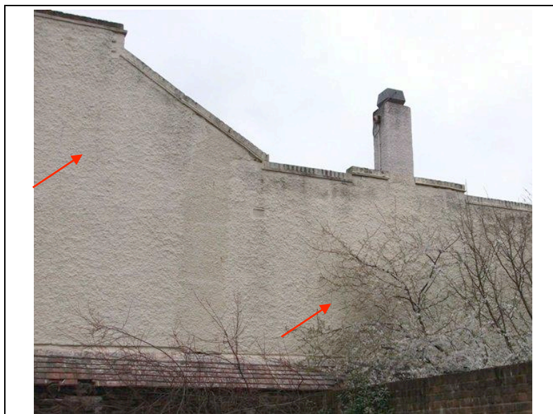
Fig. 48: Cracks to render of west elevation
