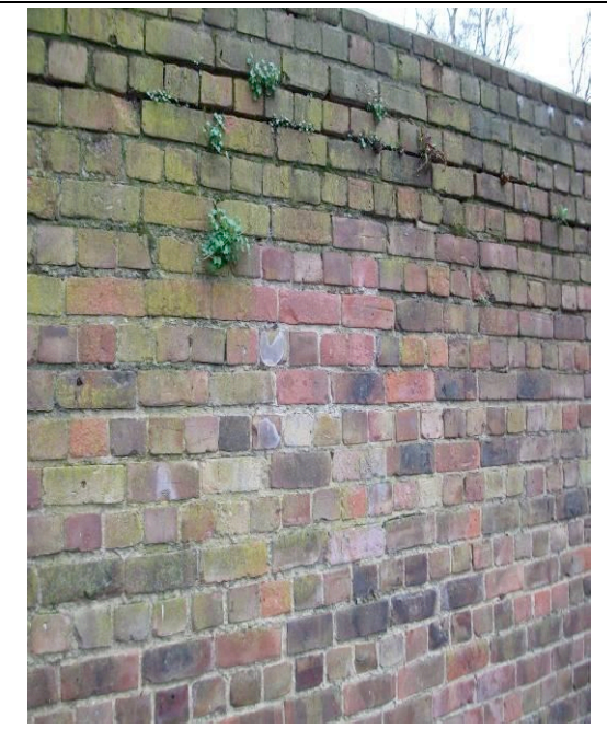
Fig. 13: A section of the wall from the car park showing loss of pointing, biological growth and a recent repair.
