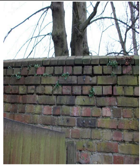
Fig. 11: A section of the wall from the Car Park side showing serious loss of pointing.
